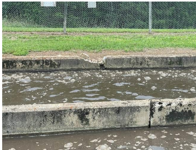
8 9 Crack in concrete tank at Chelsea Rose facility with signs of leaking
