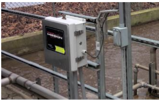
Newly installed remote monitoring system
