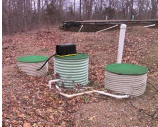
Micro MBBR in Recirculation tank and small blower running MBBR at Cimarron Bay
