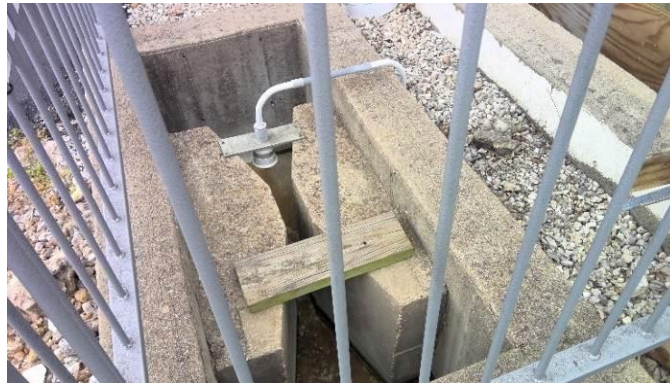
7 8 Ultrasonic Flow Meter at Cedar Green
