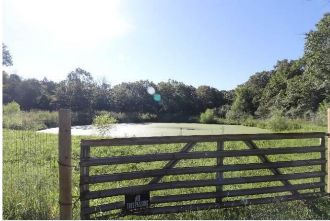
Overgrowth around lagoon, varmint damage on berms visible
