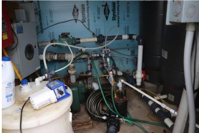
4 Well house interior, note coils of garden hose, rusted well head plate, exposed wiring, bleach bottle
