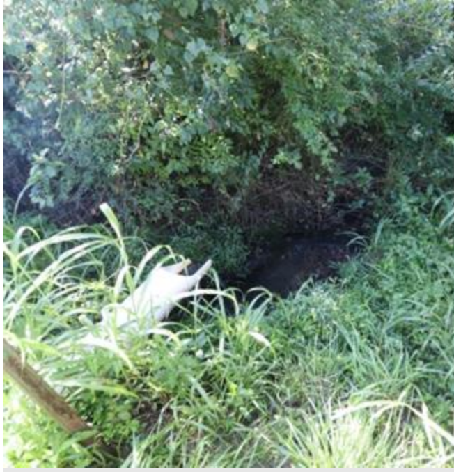
Discharge from single cell lagoon with no disinfection equipment
