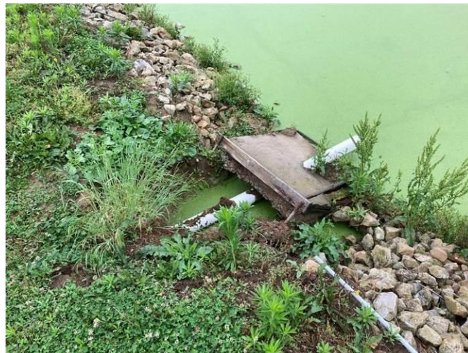
Erosion behind transfer pipe
