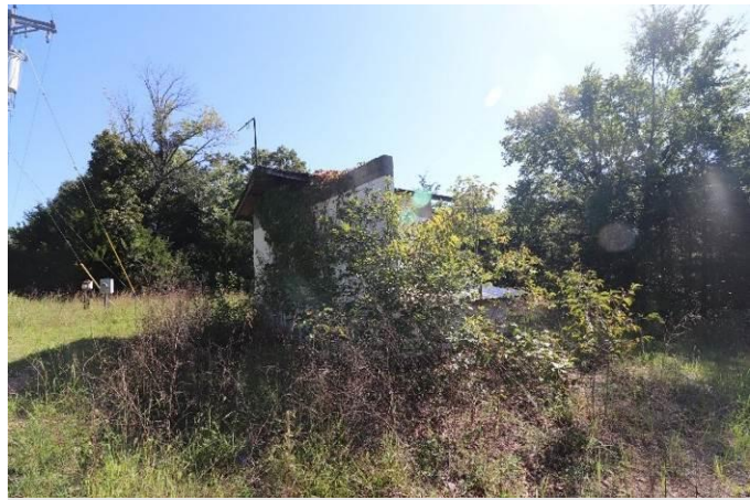
Vegetation overgrowing the Well #2 well house.
