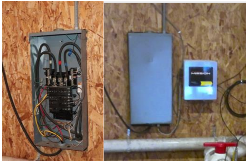
12 13 Damaged power panel, exposed wiring at Cedar Glen. Panel repaired and remote monitoring installed. 14
