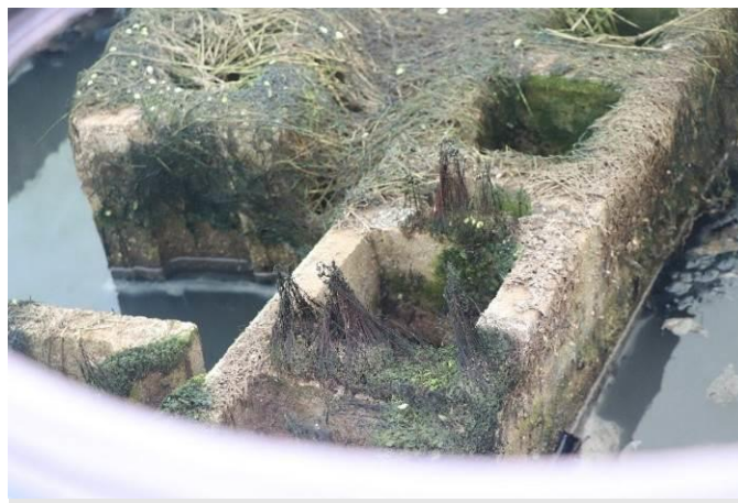
10 11 Sludge filled contact chamber with significant vegetation growth at Eagle Woods
