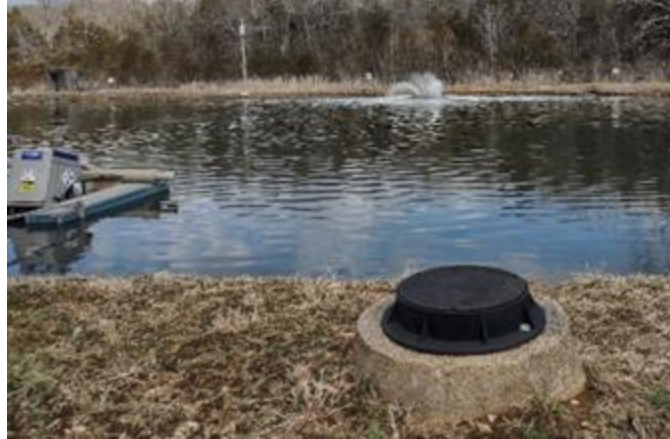
New Airmaster aerators installed in first cell of the lagoon system
