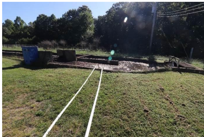
Above ground RAS lines at Oxidation Ditch
