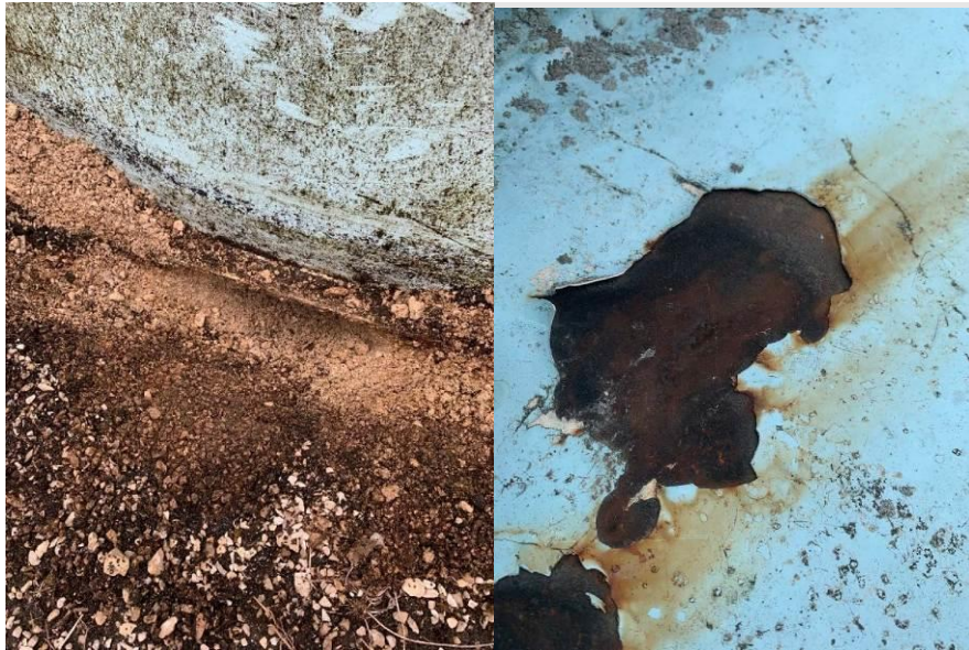
3 4 Erosion around standpipe gravel footing / corrosion to standpipe coating 5 6
