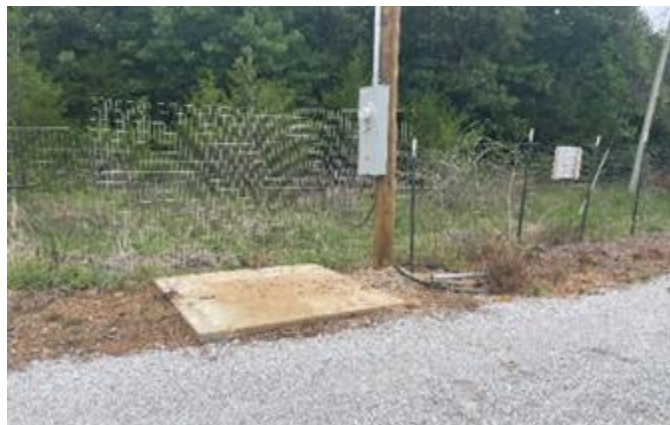
Site of old control shack and new power service to site
