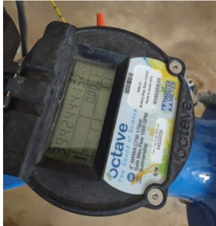
New Flow Meter at well #4
