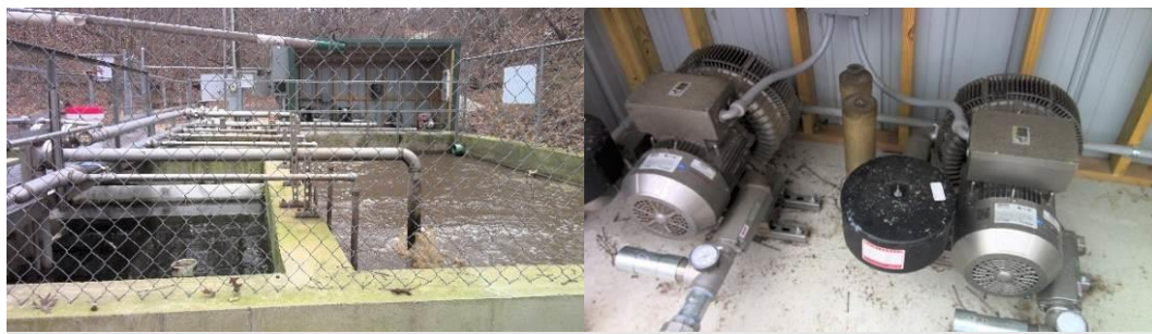
New aeration piping, blowers, and valving
