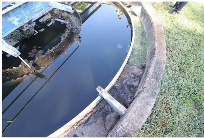
7 8 Significant accumulation of sludge in skimmer trough due to failed mechanical components of clarifier 9
