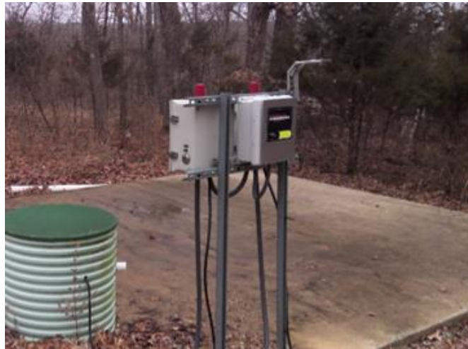
6 7 Remote monitoring unit at treatment facility
