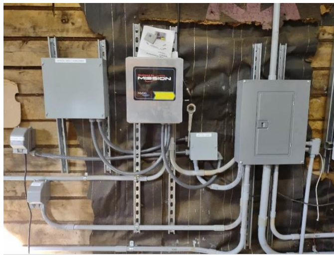
Remote monitoring installed at Well #1
