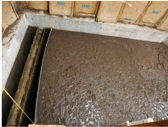
6 7 Clarifier at Cedar Green filling with pin floc sludge, indicating failed skimmers
