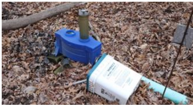
New dechlorination tablet feeder
