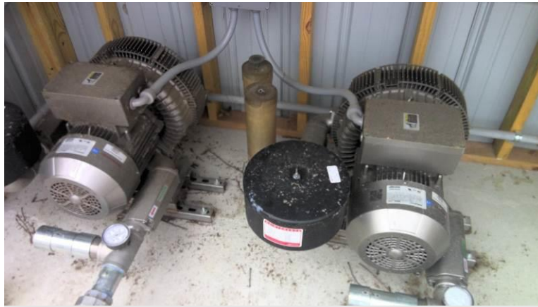
New blowers at the Chelsea Rose facility which had no functional blowers at acquisition
