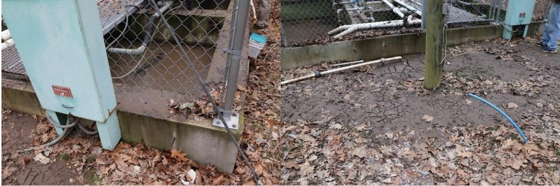
1 2 Large amounts of sludge deposited on the ground around the facility from past overflow, signs of recent 3 overflow with wet sludge on the top edges of the facility tankage. Also note poor piping practices with flex 4 hoses attached with hose clamps on sludge return lines rather than proper plumbing returns 5
