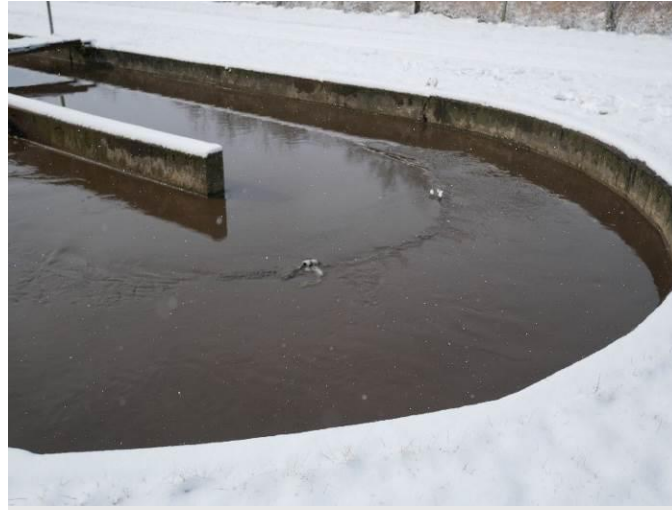
4 5 Sludge accumulation breaking the surface of water in the Oxidation Ditch
