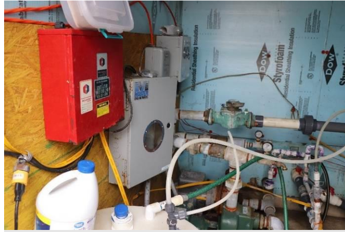
Power and control system condition at acquisition
