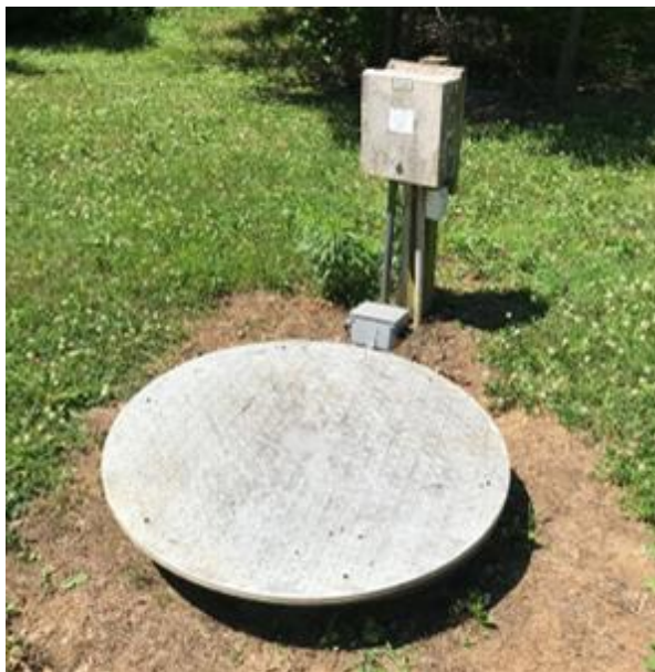
Lift station at Park Estates, missing redundant pump
