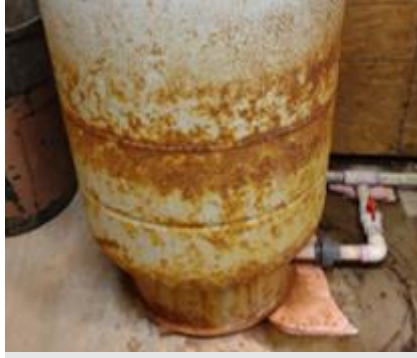
Rusting bladder tank at Missing Well system
