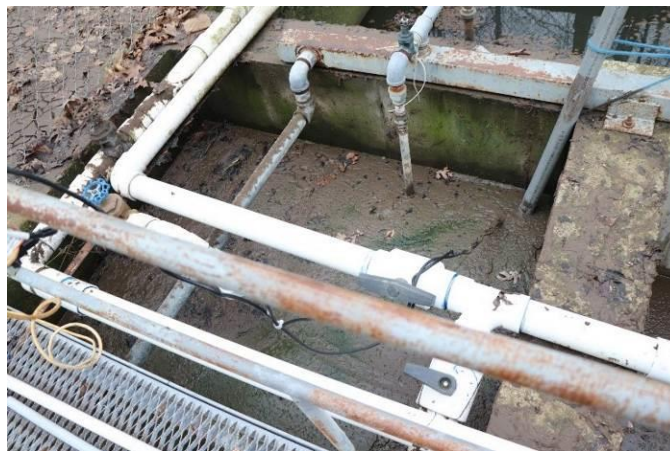
Overfilled sludge digester
