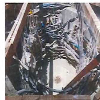
Highly congested manhole on 7 th St.
