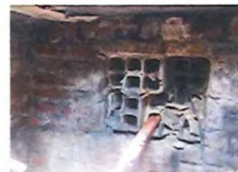
Clay tile duct bank in disrepair (still in use with existing fiber)
