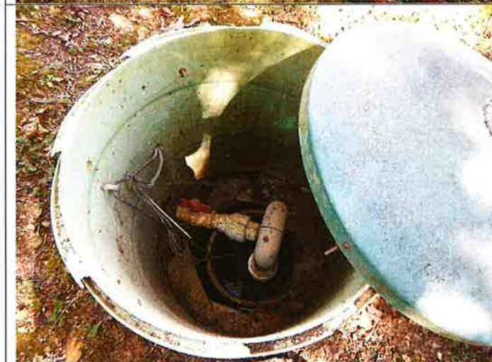
Photograph #: 012 Taken by: Elizabeth Stephens Entity: Confluence Rivers-Port Perry WWTF Permit: MOG823126 Location: Perry County Description: Inside view of lift station. Date Taken: October 1, 2020 Program: WPC Unit
