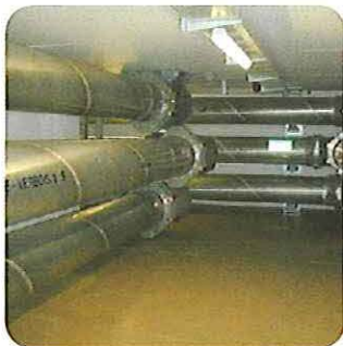
GIL installed in tunnel.
