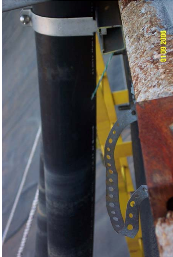
Figure 5.6 - High Water marks on HDPE Tubes
