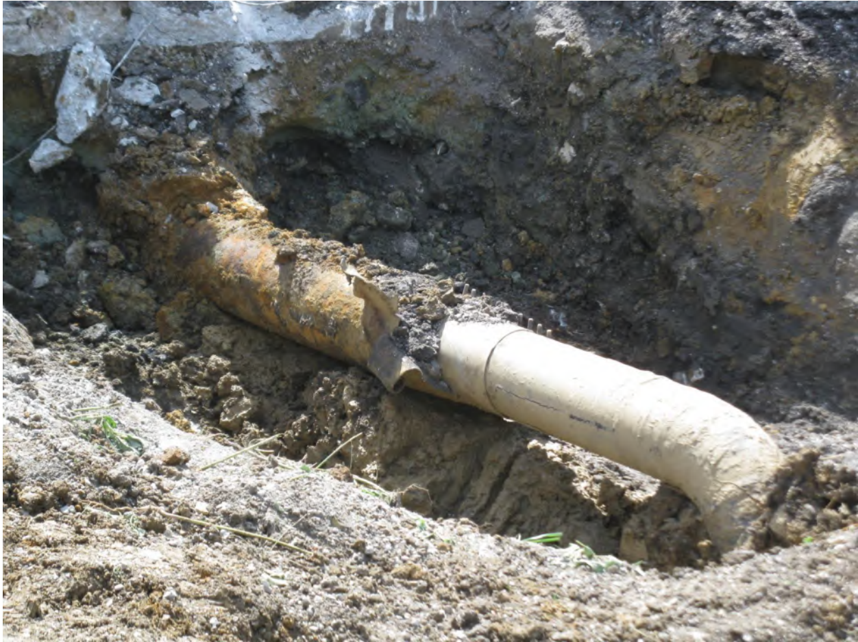
Photograph 4: Photograph of the damaged portion of the pipeline looking southeast. A repair clamp is surrounding the damaged portion of the pipeline. (Source: Staff)
