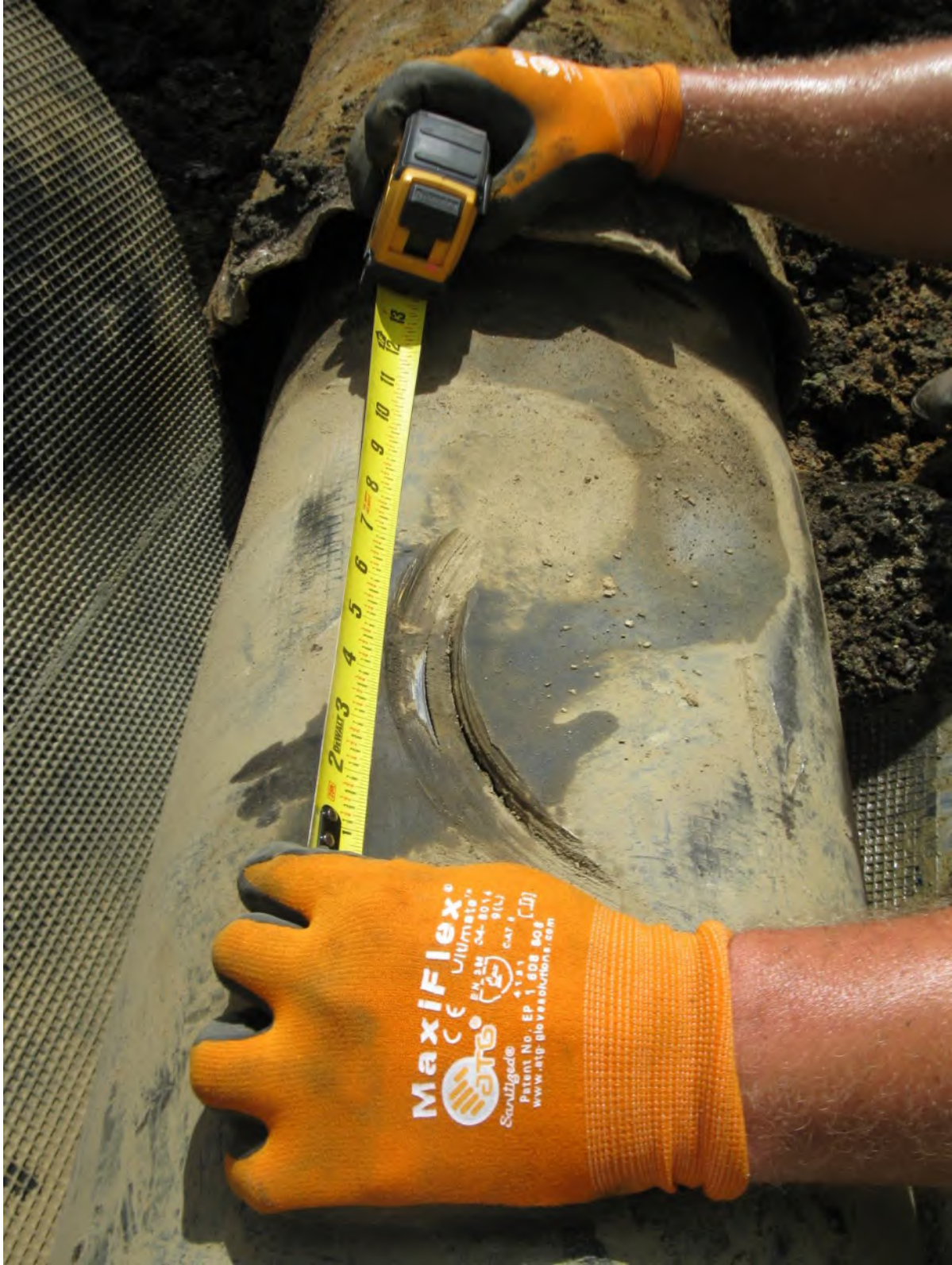
Photograph 6: Photograph of the damage to the pipeline. (Source: Staff)
