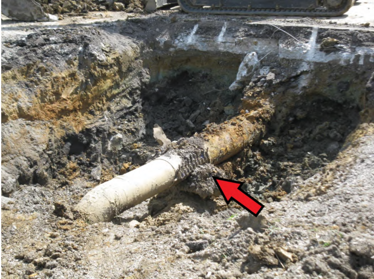
Photograph 3: Photograph of the damaged section of pipeline looking northeast. The red arrow (added by Staff) points to a repair clamp surrounding the damaged portion of the pipeline. (Source: Staff)
