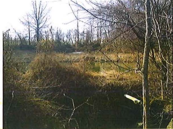
Old Lagoon with Illegal Untreated Drain
