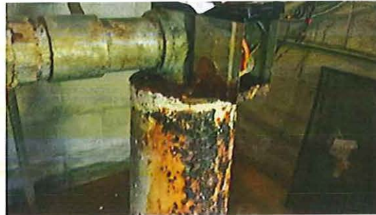
Corroded Hillcrest Drinking Water Well Head
