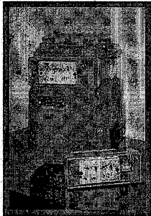
Automated Meter Reading
