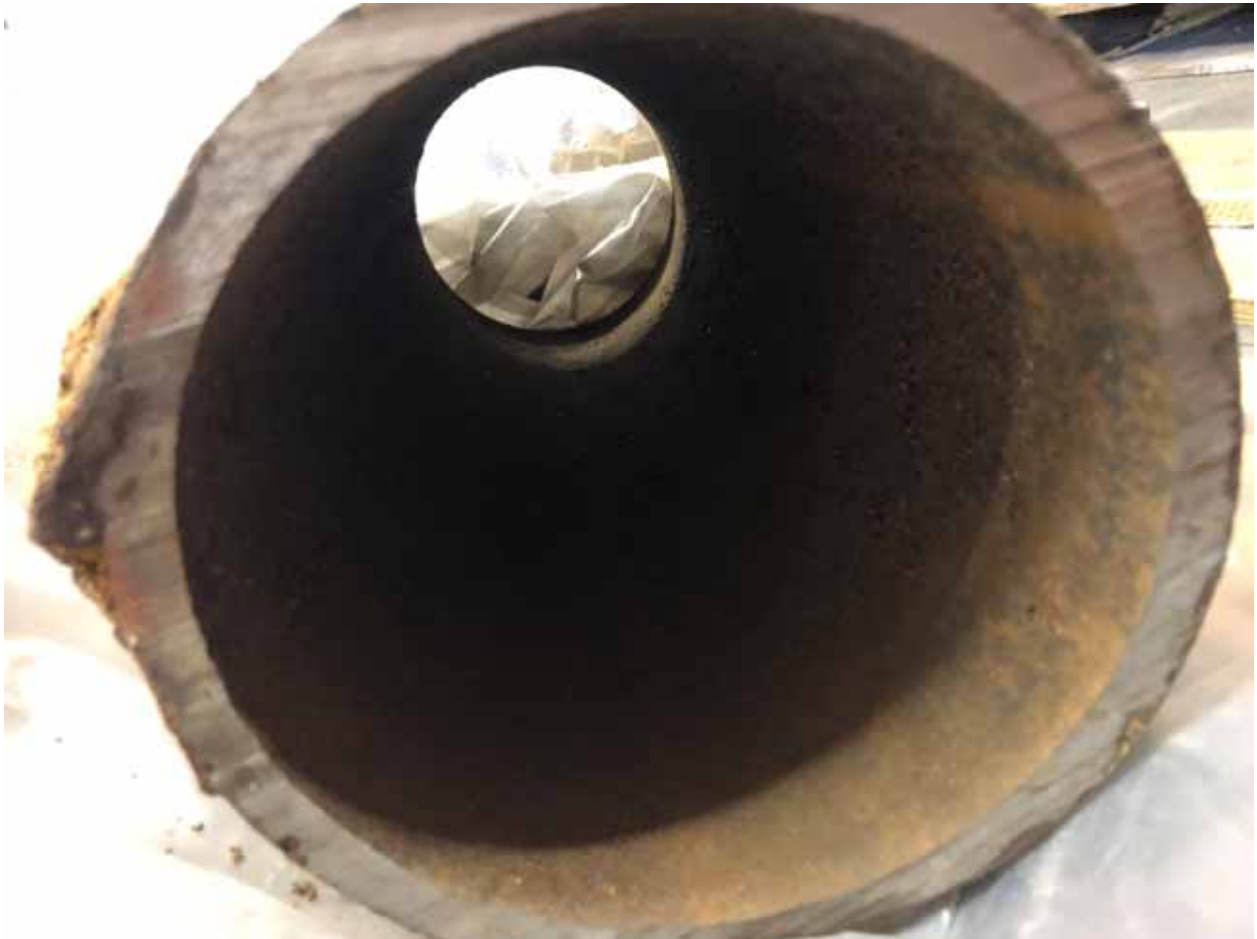
Figure 7, Spire East, North Region, Cast Iron, Work Order #18698297
