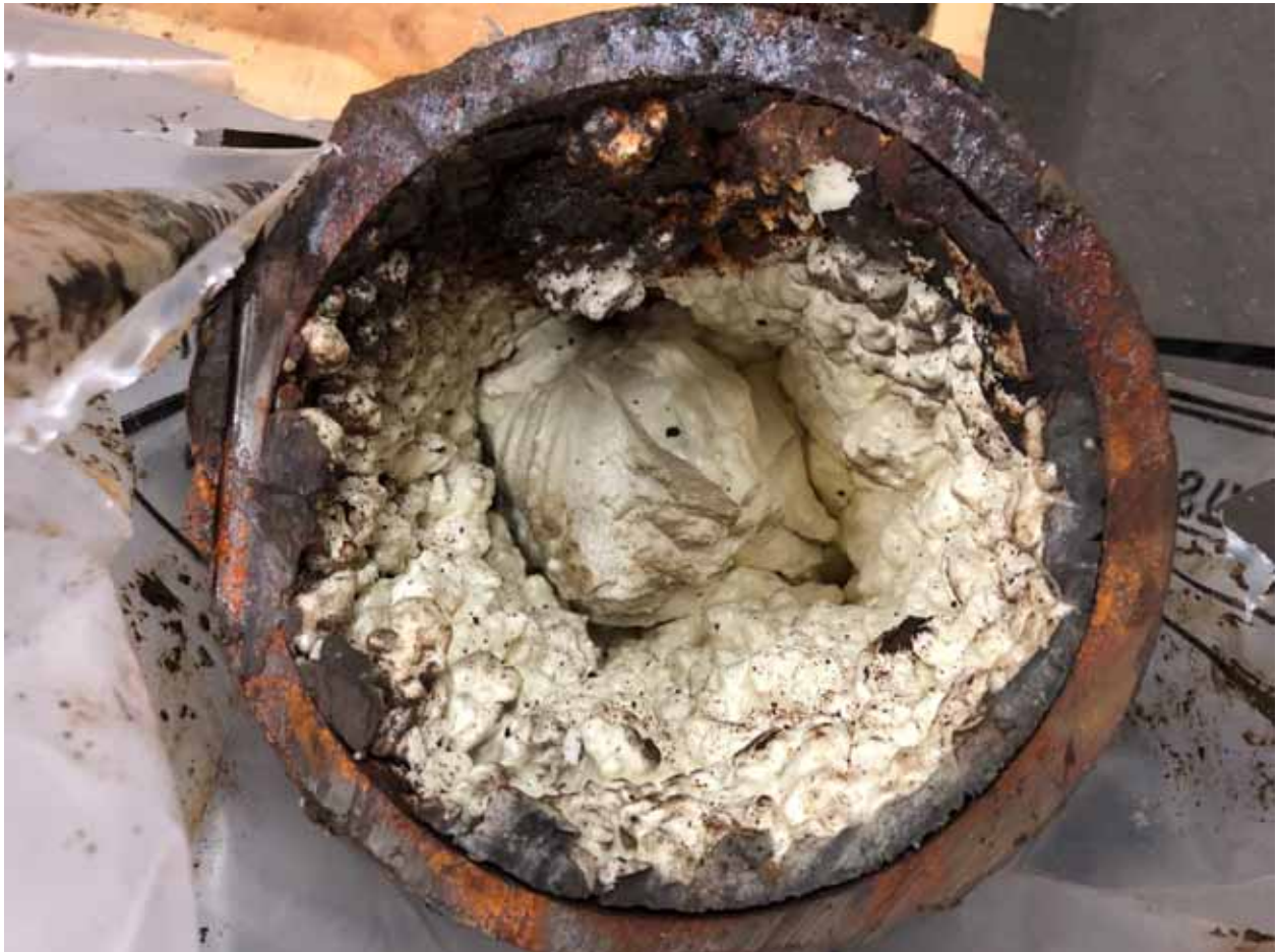
Figure 14, Spire East, North Region, Cast Iron, Work Order #18899931
