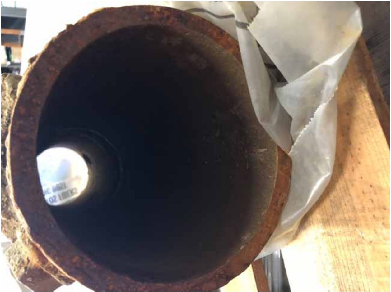
Figure 2, Spire East, North Region, Cast Iron, Work Order #83698313
