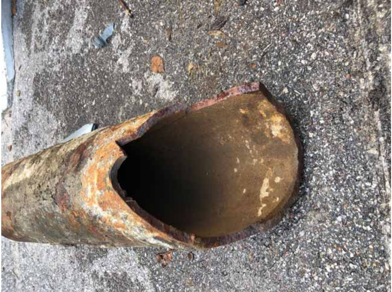
Figure 36, Spire East, South Region, Cast Iron, Work Order #19655345
