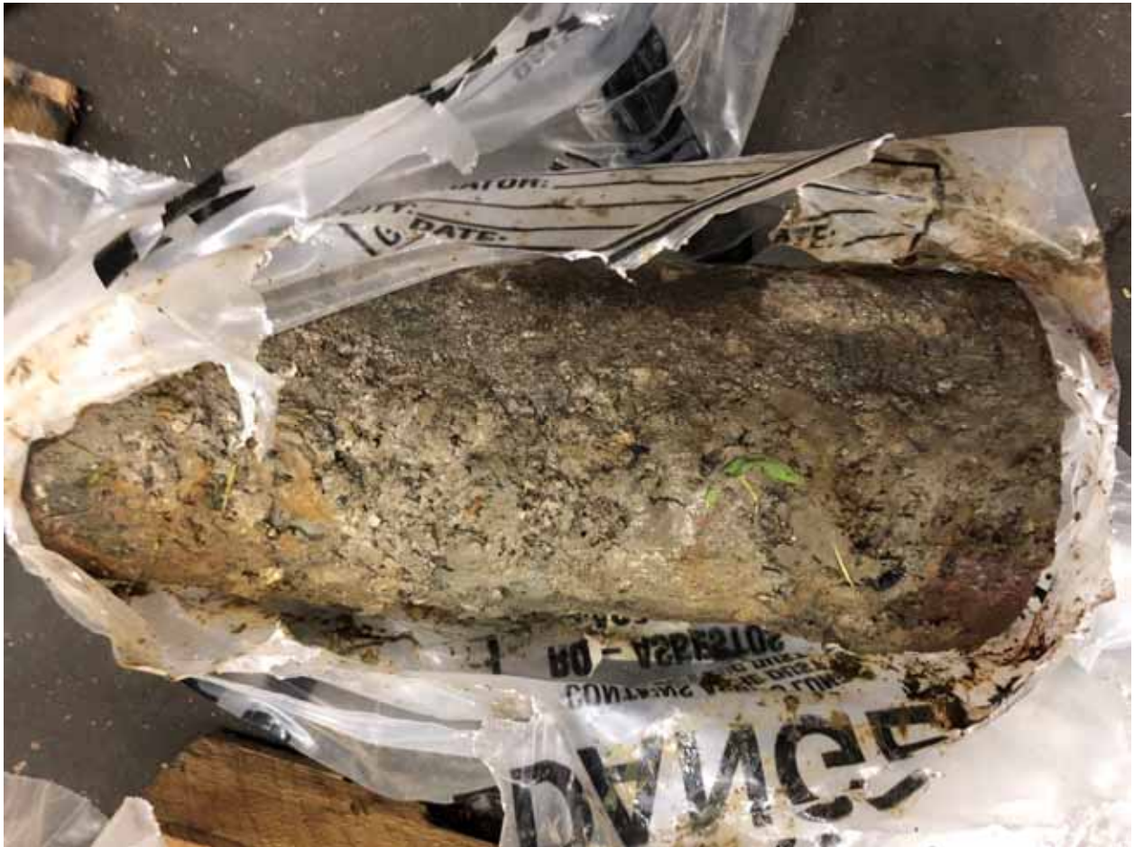
Figure 13, Spire East, North Region, Cast Iron, Work Order #18899931
