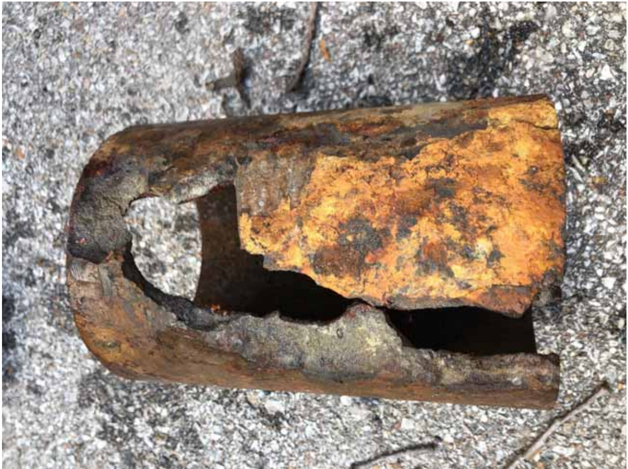
Figure 27, Spire East, South Region, Cast Iron, Work Order #171733652
