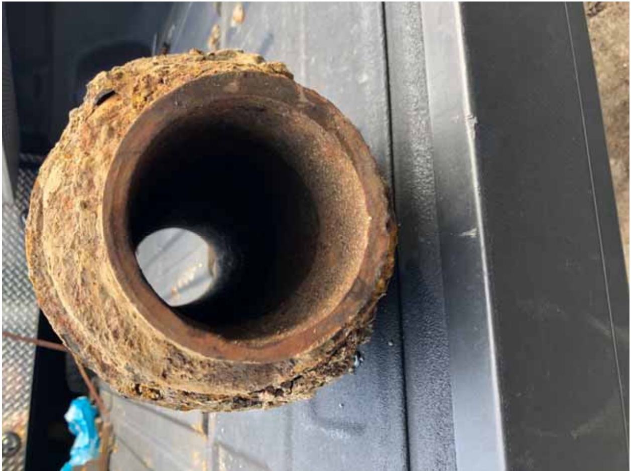
Figure 43, Spire East, South Region, Cast Iron, Work Order #196553364
