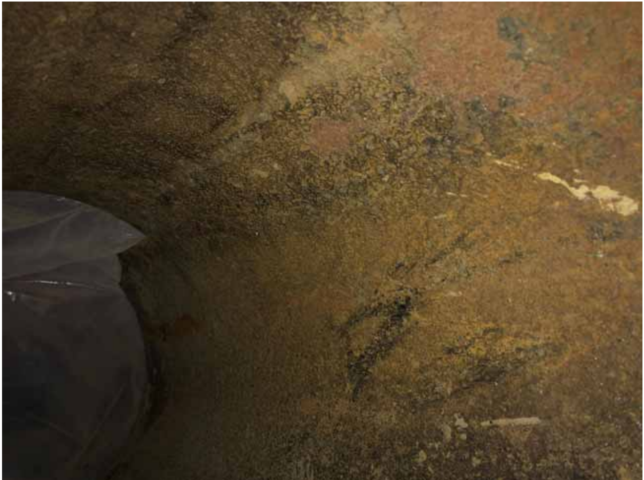
Figure 19, Spire East, North Region, Cast Iron, Work Order #20351410
