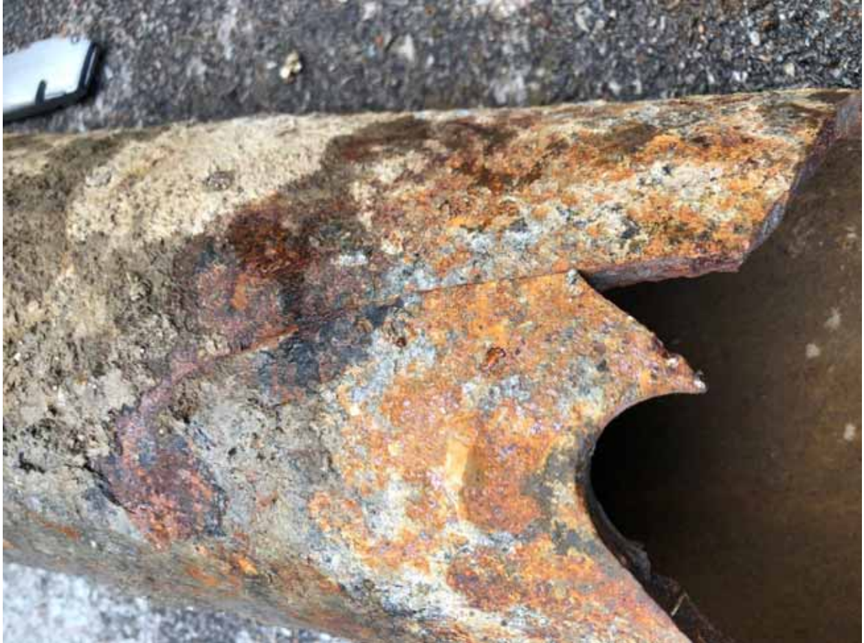
Figure 37, Spire East, South Region, Cast Iron, Work Order #19655345
