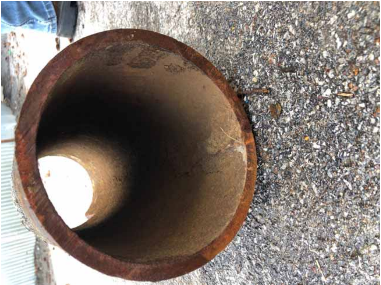
Figure 38, Spire East, South Region, Cast Iron, Work Order #19655345
