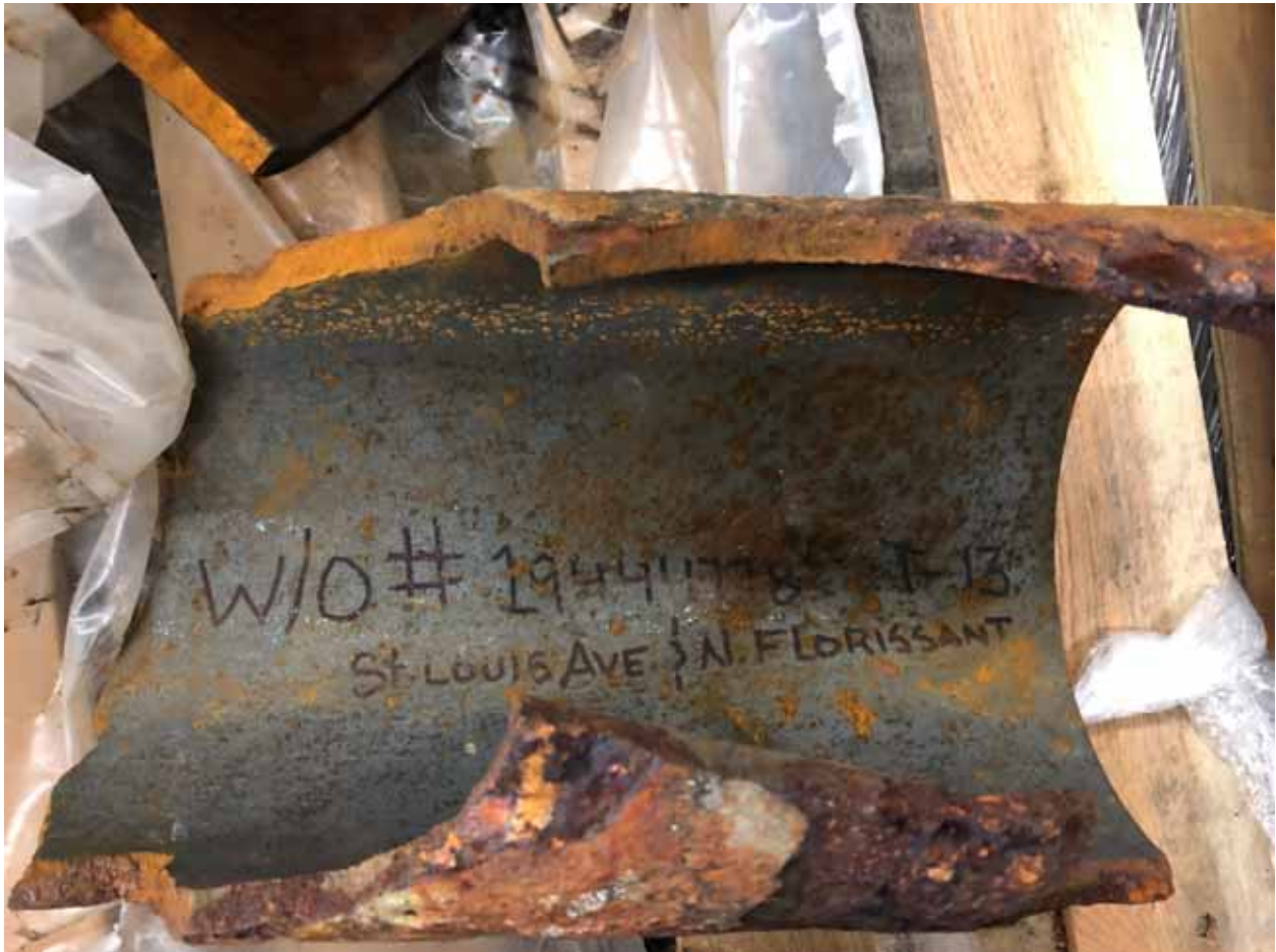
Figure 8, Spire East, North Region, Cast Iron, Work Order #19444778
