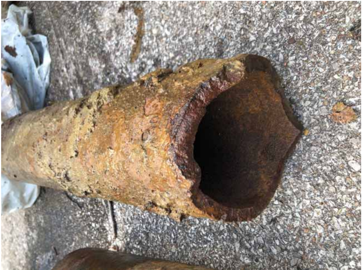
Figure 31, Spire East, South Region, Cast Iron, Work Order #171733652
