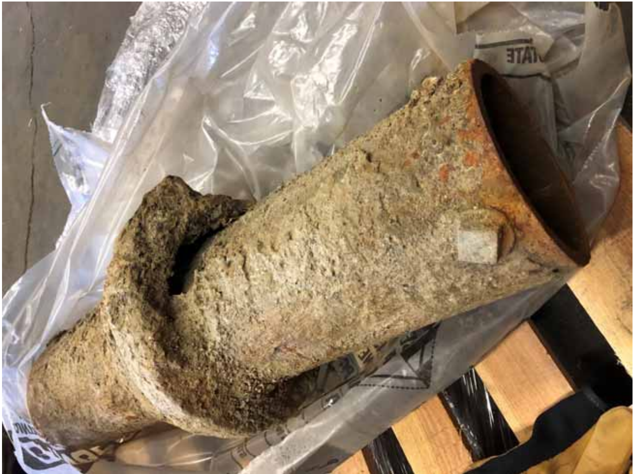
Figure 1, Spire East, North Region, Cast Iron, Work Order #83698313
