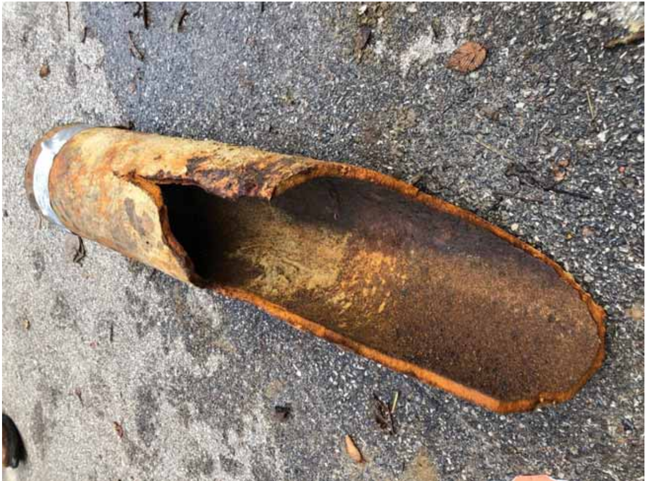
Figure 41, Spire East, South Region, Cast Iron, Work Order #15515587
