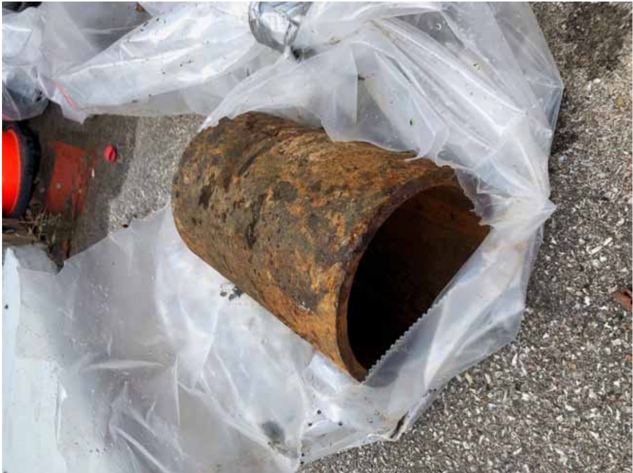
Figure 20, Spire East, South Region, Cast Iron, Work Order #19251195
