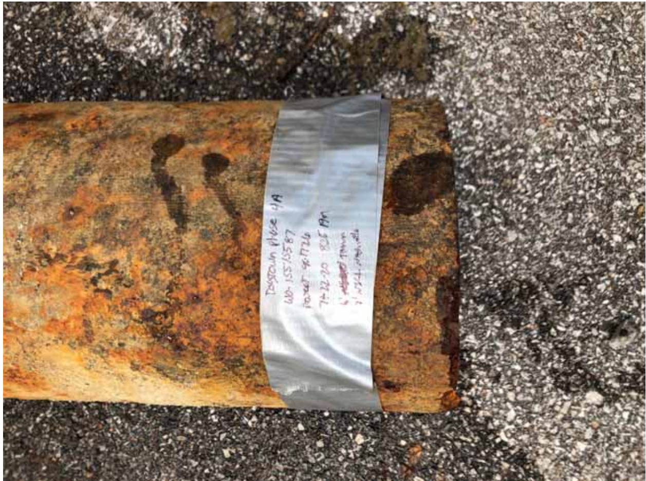
Figure 39, Spire East, South Region, Cast Iron, Work Order #15515587
