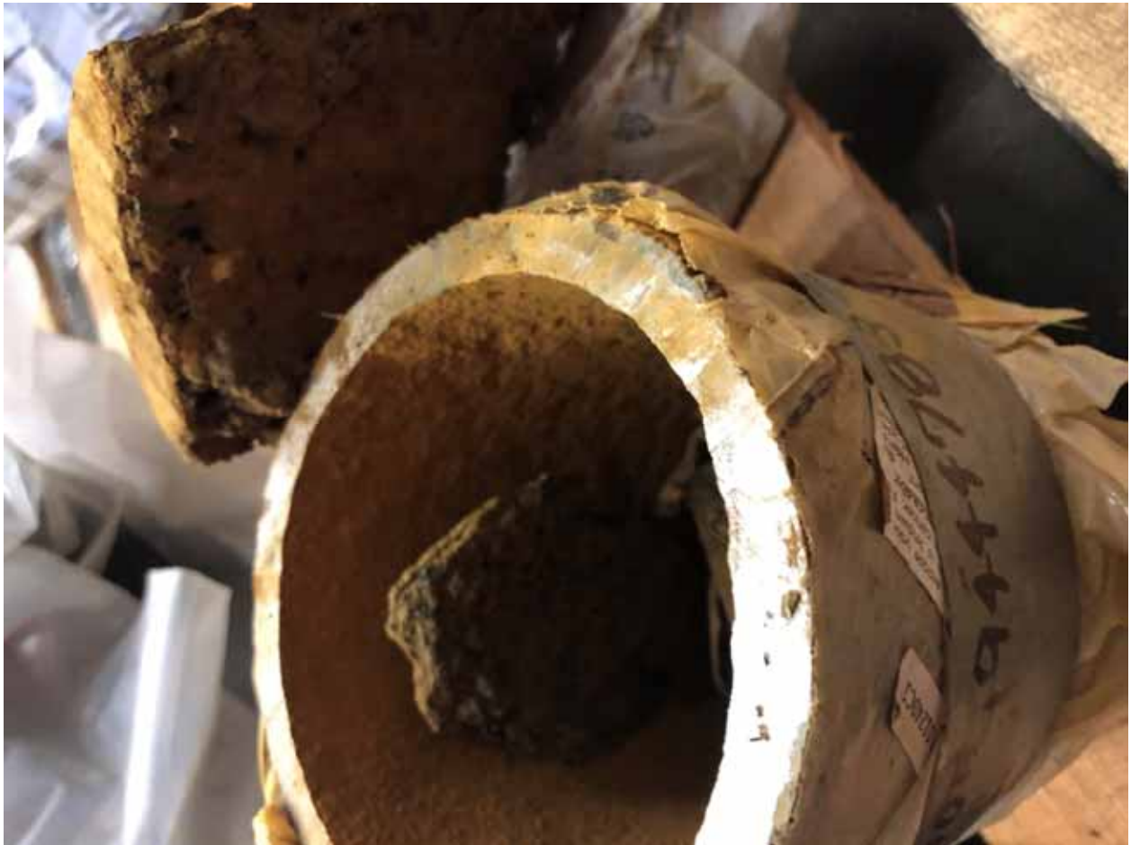
Figure 4, Spire East, North Region, Cast Iron, Work Order #19444783
