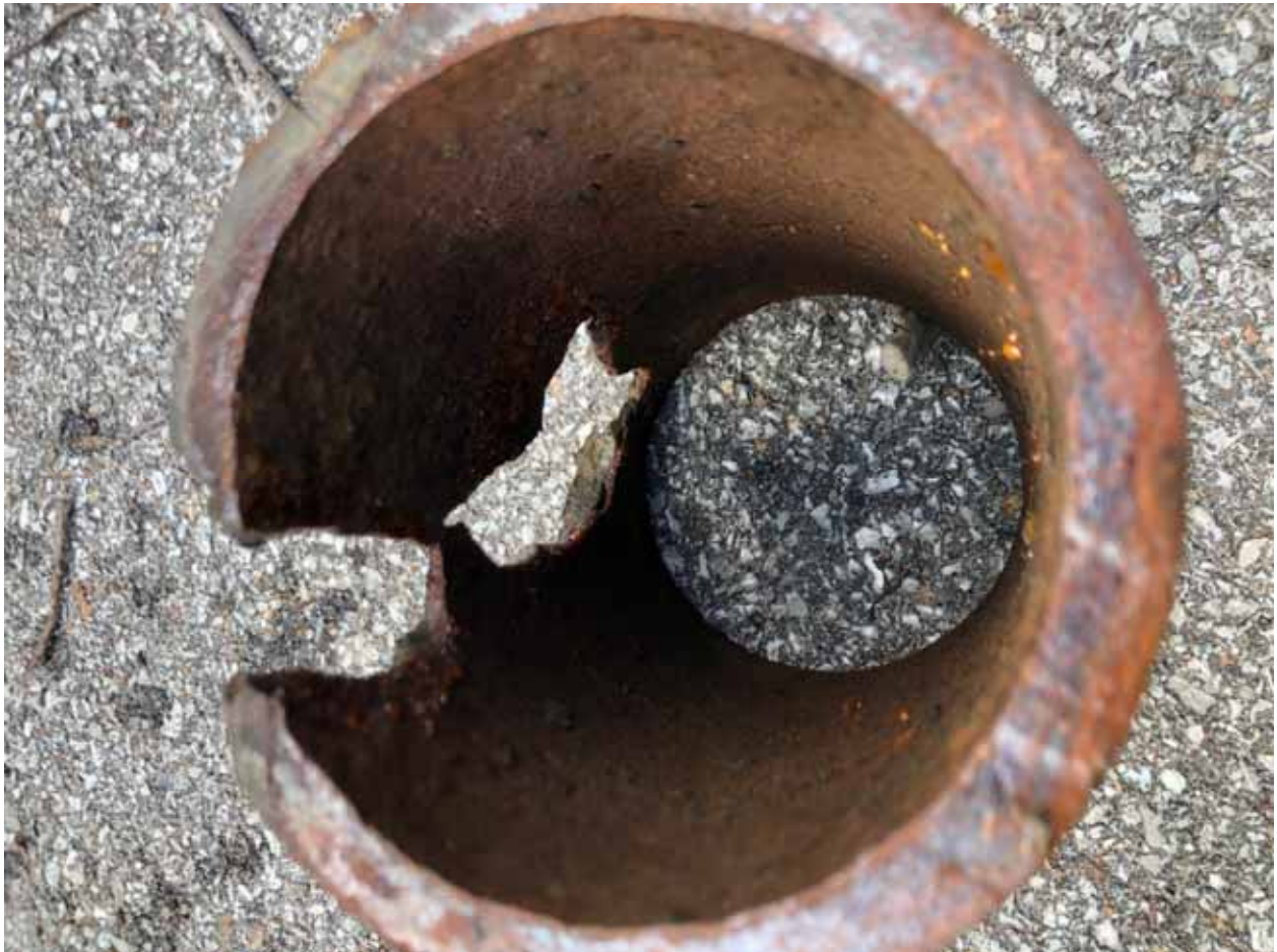
Figure 28, Spire East, South Region, Cast Iron, Work Order #171733652
