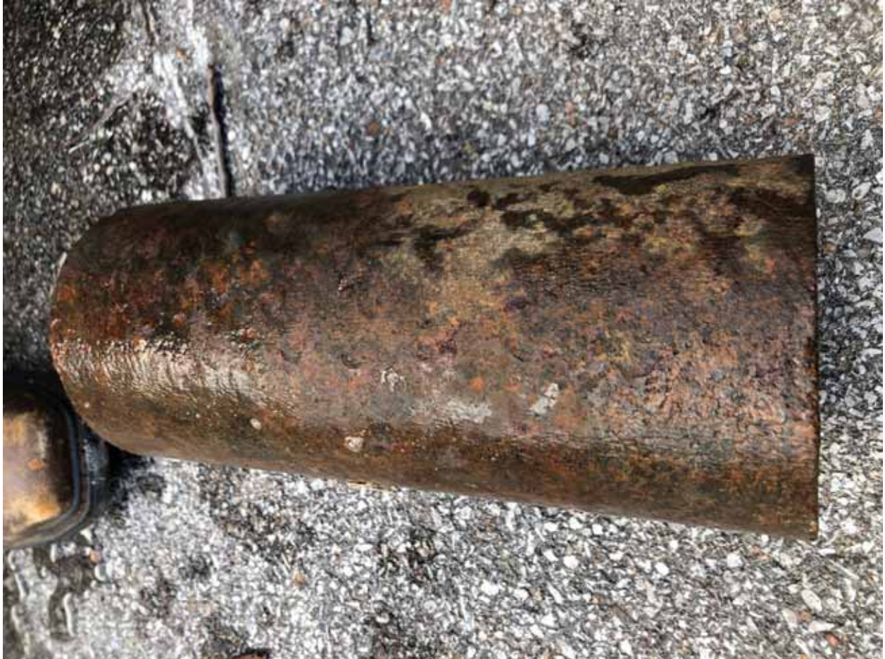
Figure 29, Spire East, South Region, Cast Iron, Work Order #171733652
