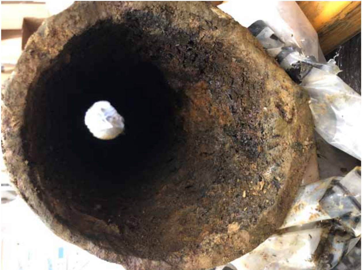
Figure 16, Spire East, North Region, Cast Iron, Work Order #20351410
