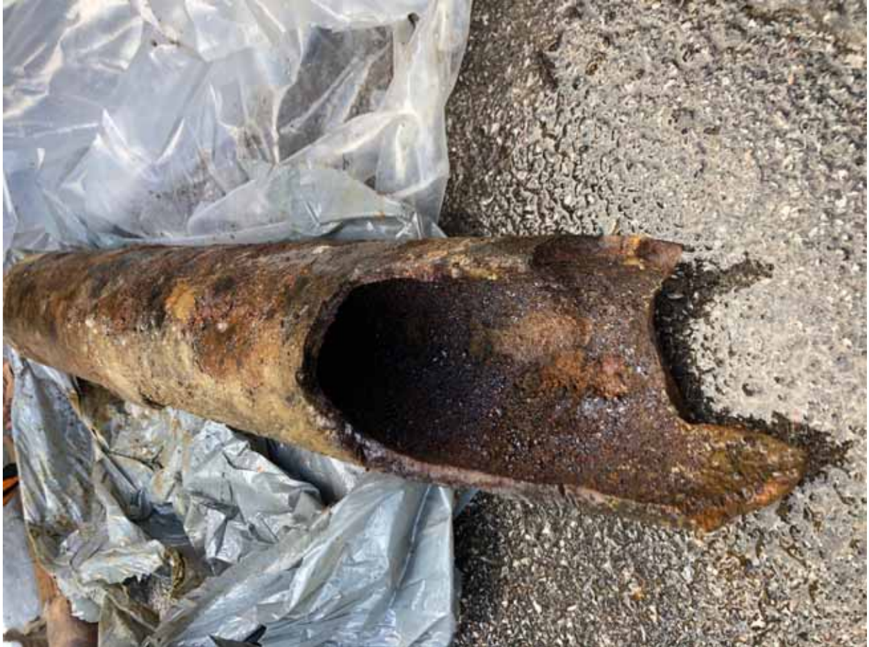
Figure 24, Spire East, South Region, Cast Iron, Work Order #20655987
