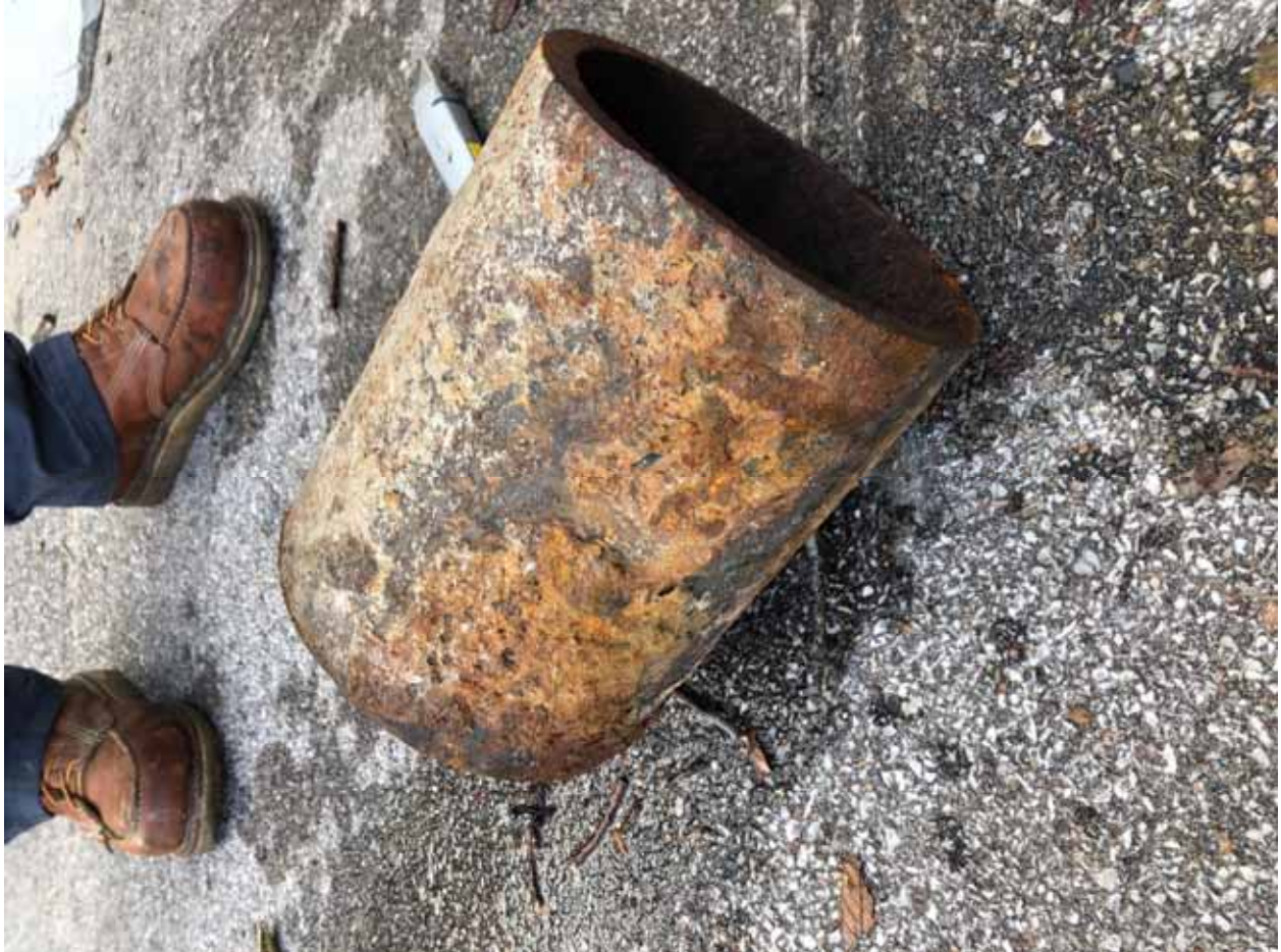
Figure 32, Spire East, South Region, Cast Iron, Work Order #17984965
