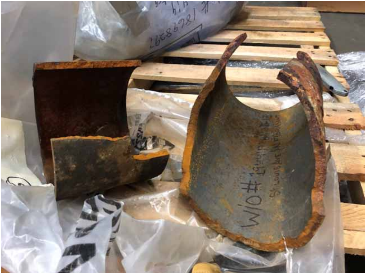
Figure 9, Spire East, North Region, Cast Iron, Work Order #18698297
