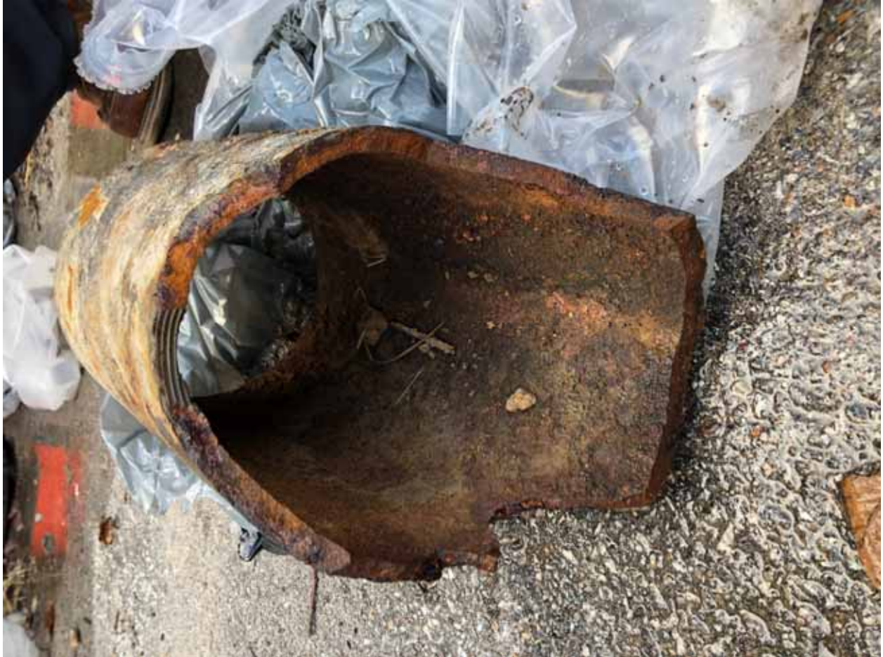
Figure 23, Spire East, South Region, Cast Iron, Work Order #19700612
