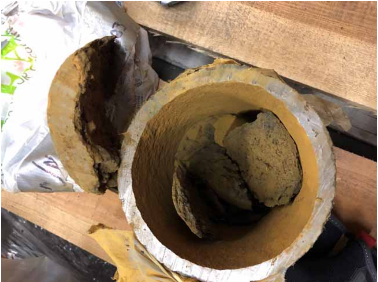
Figure 3, Spire East, North Region, Cast Iron, Work Order #19444783
