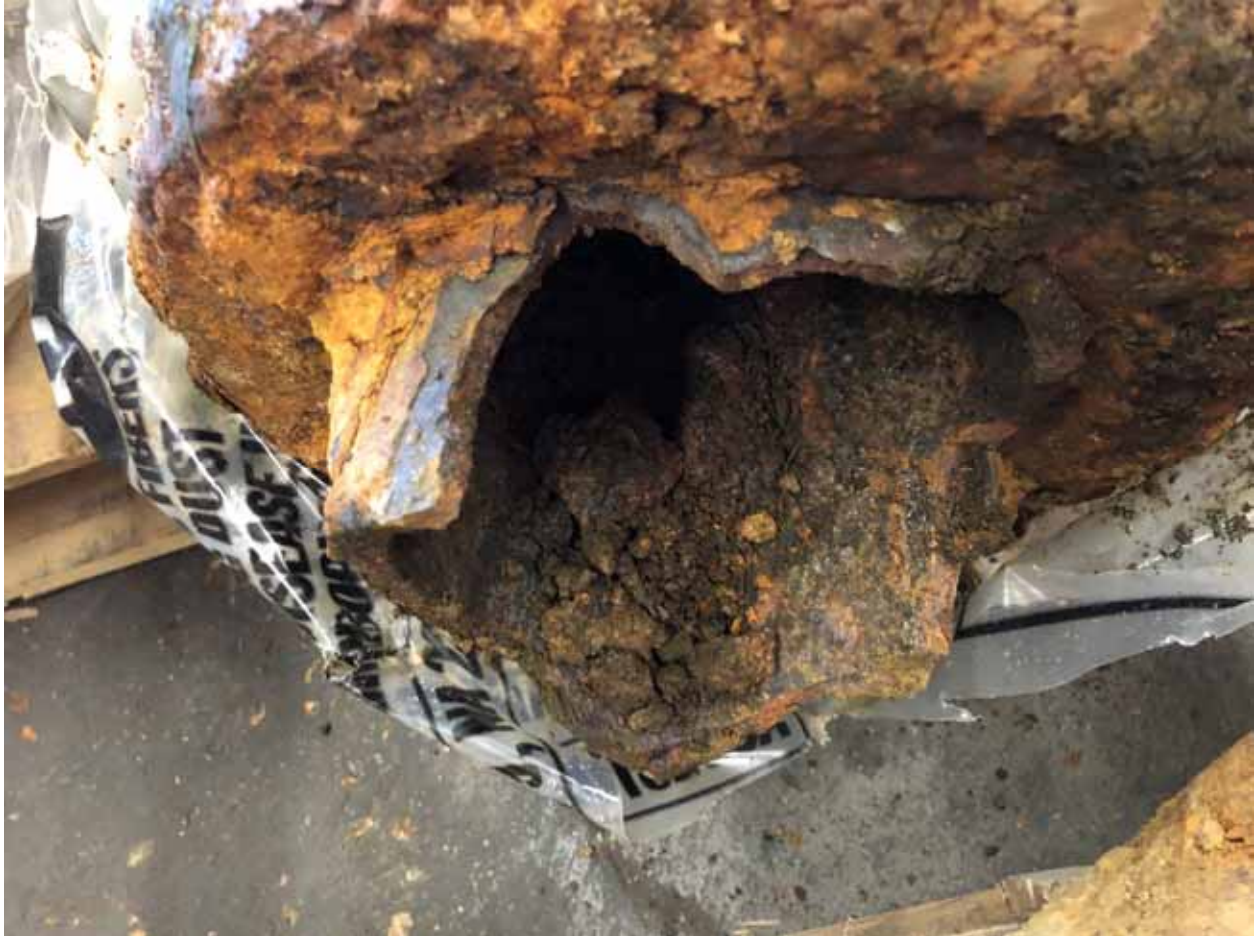
Figure 17, Spire East, North Region, Cast Iron, Work Order #20351410
