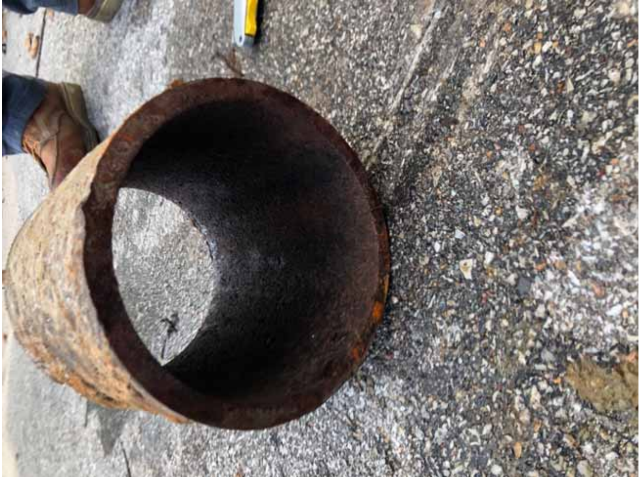
Figure 33, Spire East, South Region, Cast Iron, Work Order #17984965
