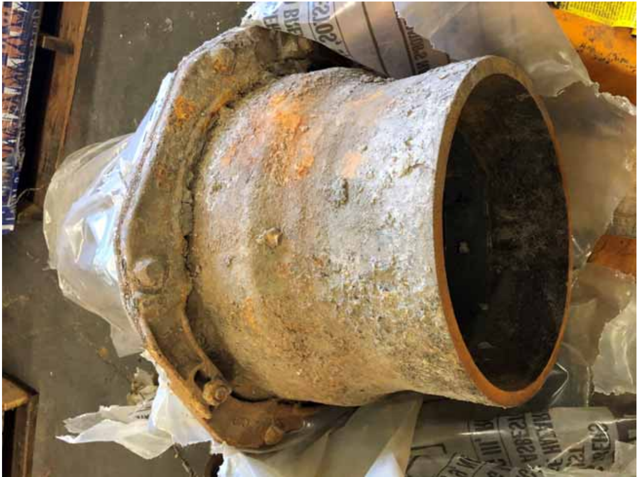
Figure 18, Spire East, North Region, Cast Iron, Work Order #20351410
