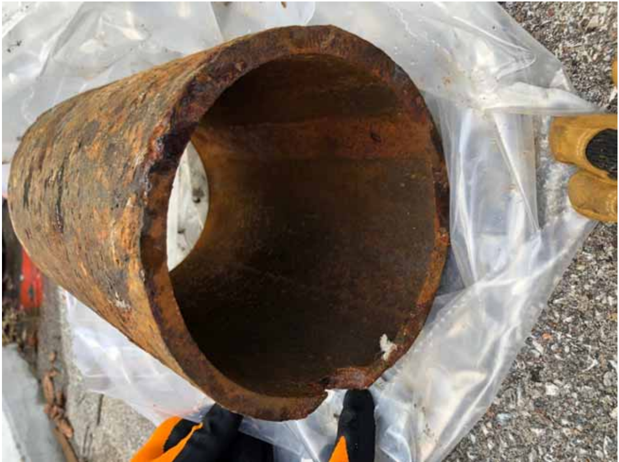
Figure 21, Spire East, South Region, Cast Iron, Work Order #19251195
