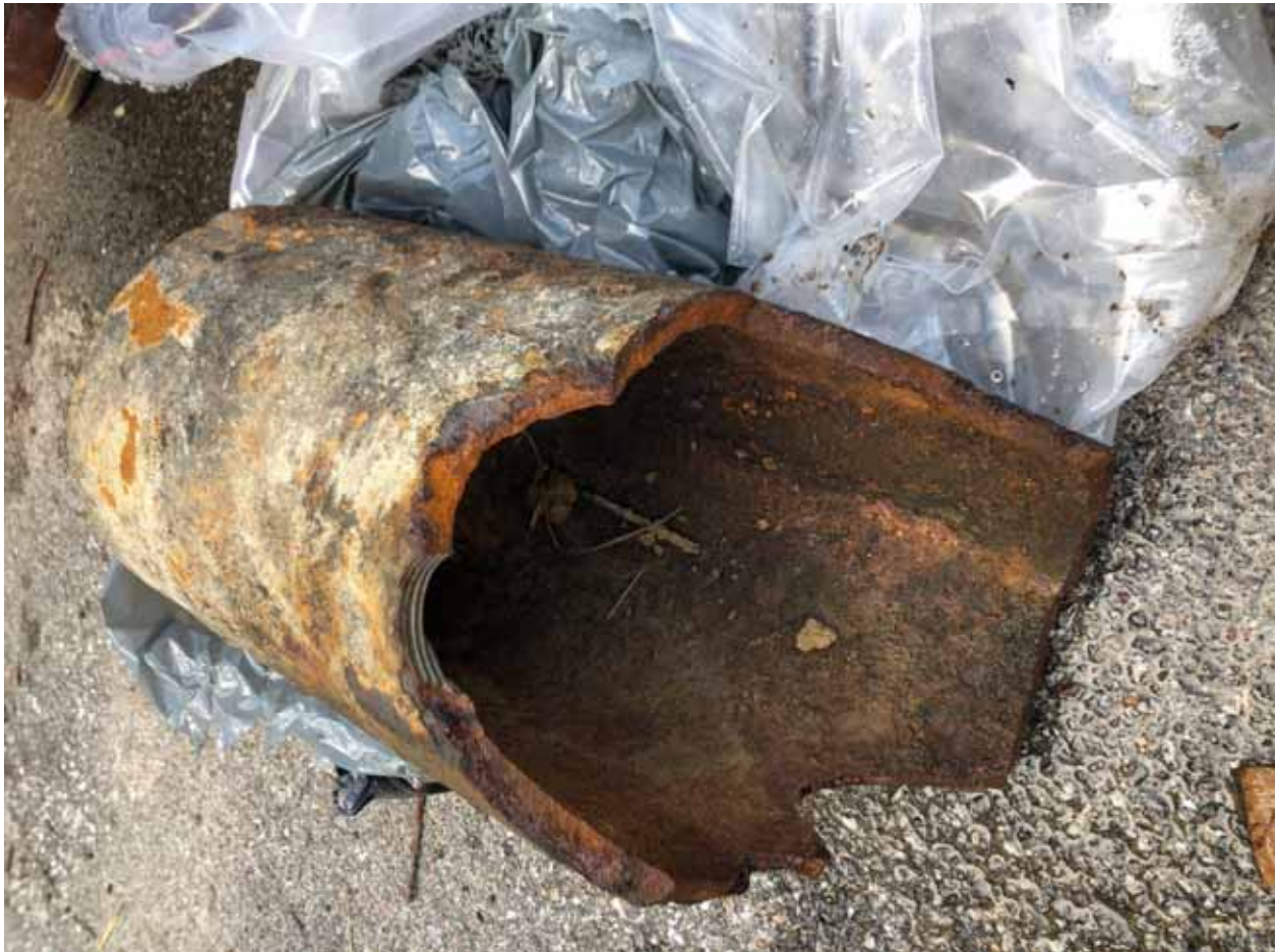
Figure 22, Spire East, South Region, Cast Iron, Work Order #19700612
