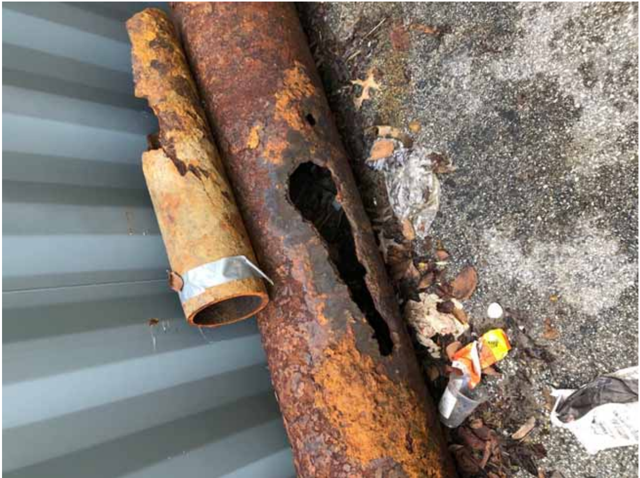
Figure 40, Spire East, South Region, Cast Iron, Work Order #15515587
