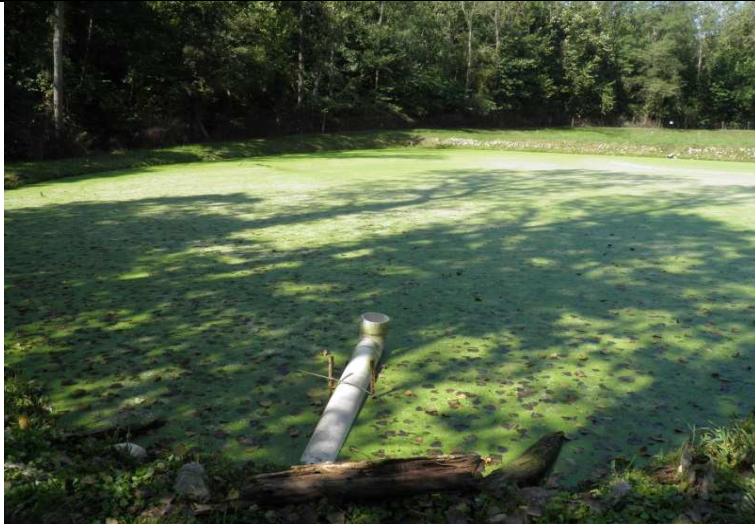
Photograph #: 4 Taken by: Stephen Moss Entity: BCSD, Trails West Subdivision Permit: #MO-0092002 Location: BOONE Description: View of the secondary cell. The outfall pipe can be observed at the bottom of the picture and a T-fitting can be observed on the influent end of the outfall pipe. Date Taken: September 1, 2016 Program: WPC Unit
