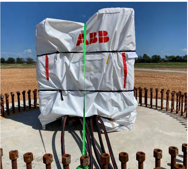
Switchgear set at T-29
