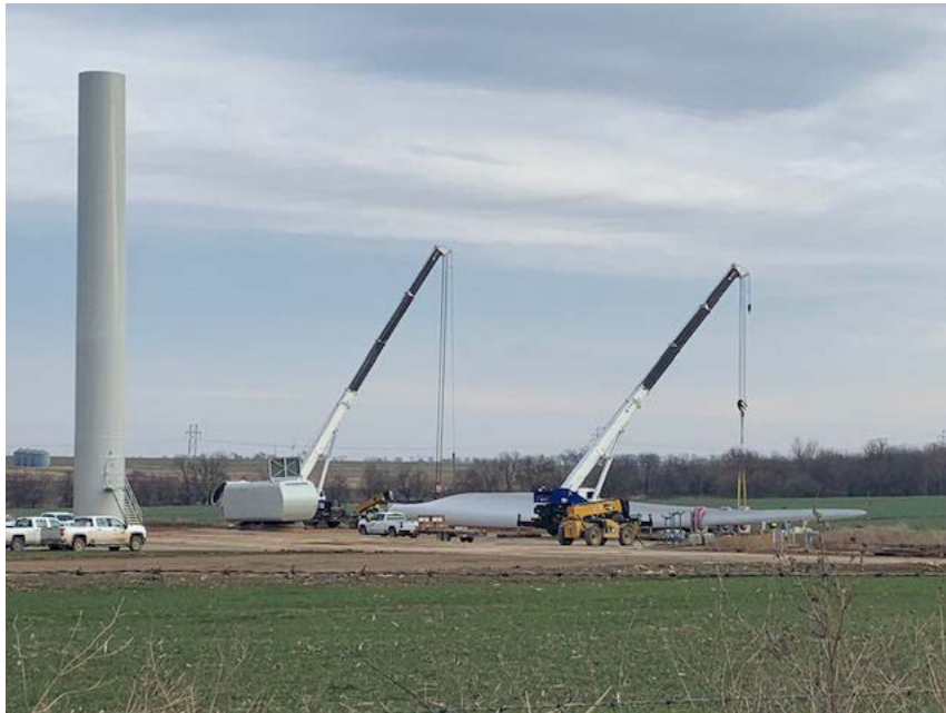
Picture 1. Offloading a turbine blade near the end of the delivery sequence.
