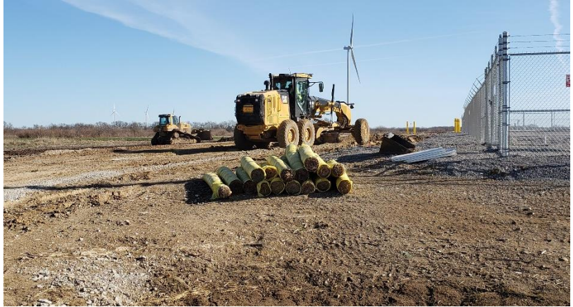
Substation & Erosion Control Blankets
