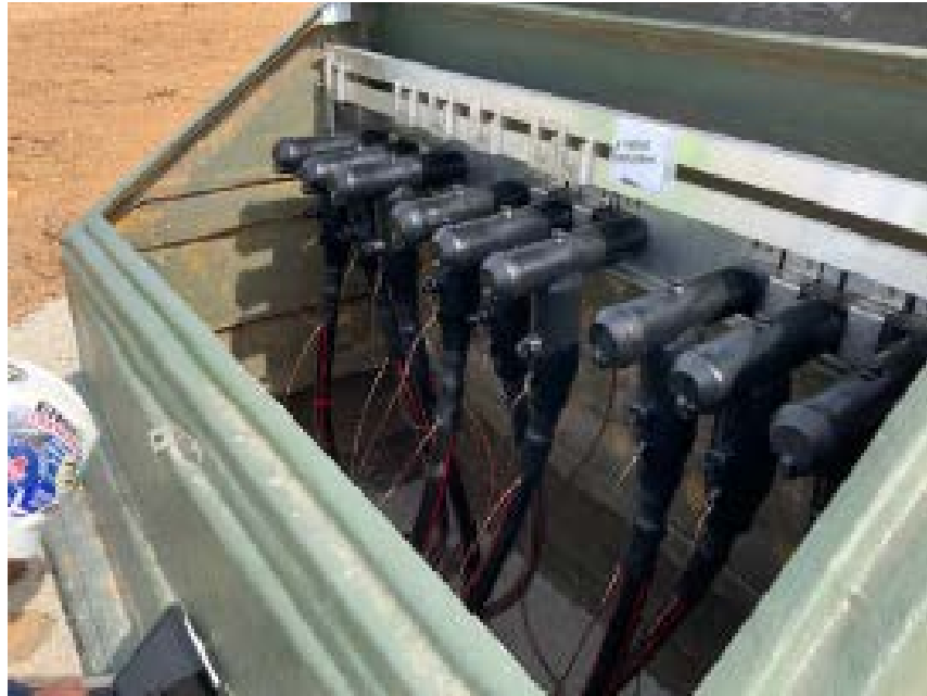
Picture 1. Collection cable terminations in a junction box.
