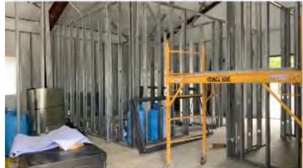
Figure 10.2: O&M Building Interior
