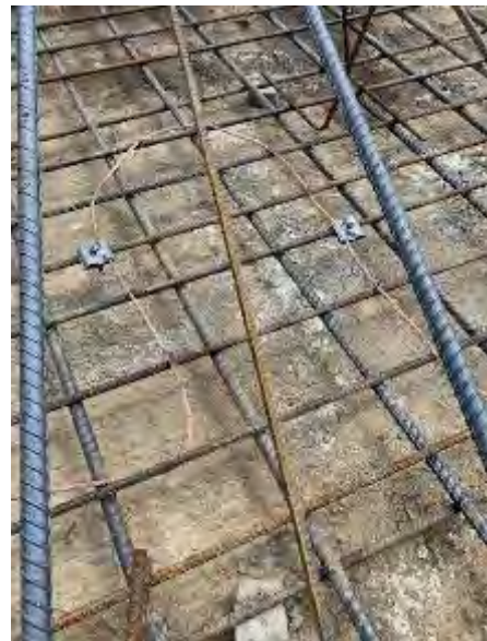
Figure 5.10: T91 Bottom Mat Grounding
