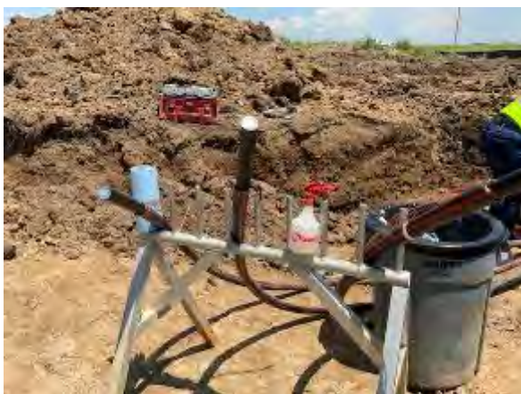
Figure 7.5: Splice Pit at T50
