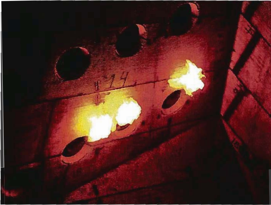
4. First fire. Burner igniters ran on natural gas for the first fire of the steam generator on November 8, 2007. Also note the near-horizontal spiral-wound "water wall" tubes in the furnace. Courtesy: Wisconsin Public Service Corp.
