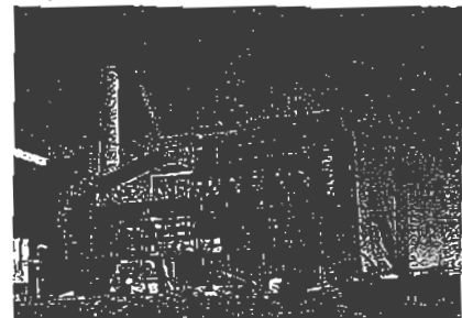
4. Raise the roof. Erection of the boiler and steel frame nearing completion. Courtesy: Hitachi
