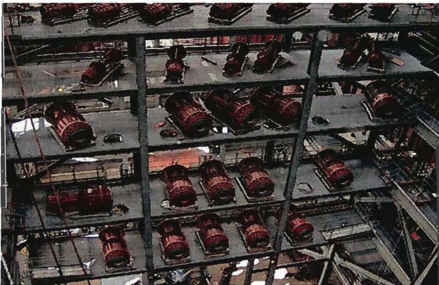
5. Ready for installation. B&W DRB-4Z low-NO x burners are staged during construction at a location that will become the furnace face. Courtesy: Wisconsin Public Service Corp.
