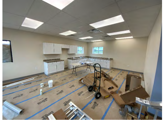
O&M Building Cabinets
