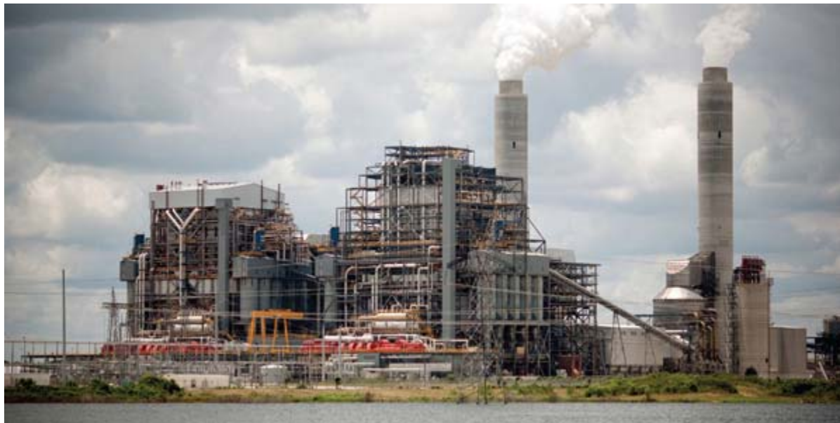
2. The odd couple. Oak Grove's Unit 1 boiler was supplied by Combustion Engineering (now Alstom Power) and the Unit 2 boiler, relocated from another project site, was supplied by Babcock & Wilcox. Courtesy: Luminant, photo by Allison V. Smith
