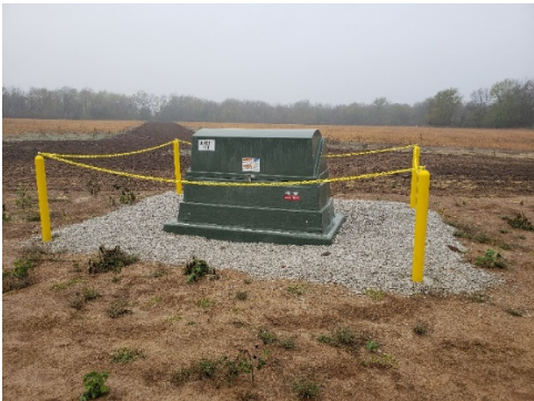
MV Cabling Box
