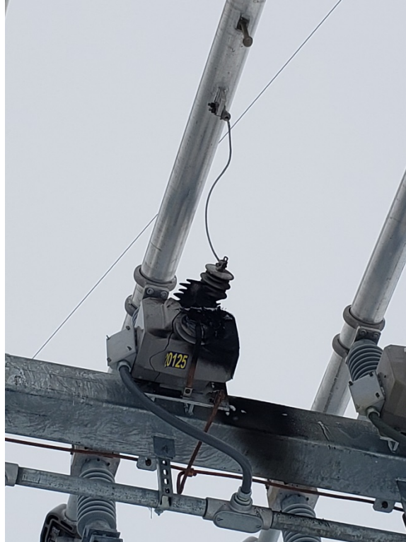
Picture 3. Failed voltage transformer at the Kings Point substation.
