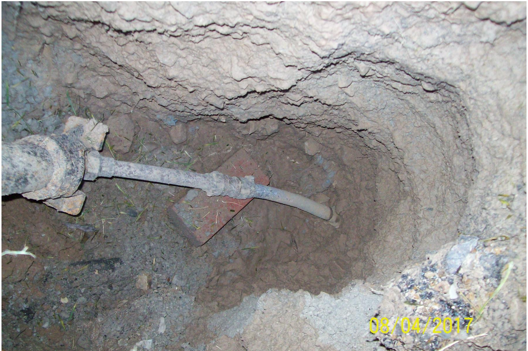
This picture shows a customer's service line that MAWC has exposed during a water main replacement. MAWC exposed the customer's service line to verify if it is lead. On the left is a short piece of copper which is then connected to a lead service line.
