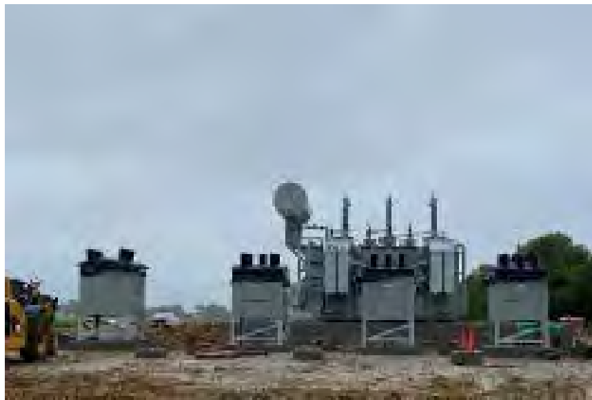
Picture 2. 34.5 kV circuit breakers in place at collector substation.
