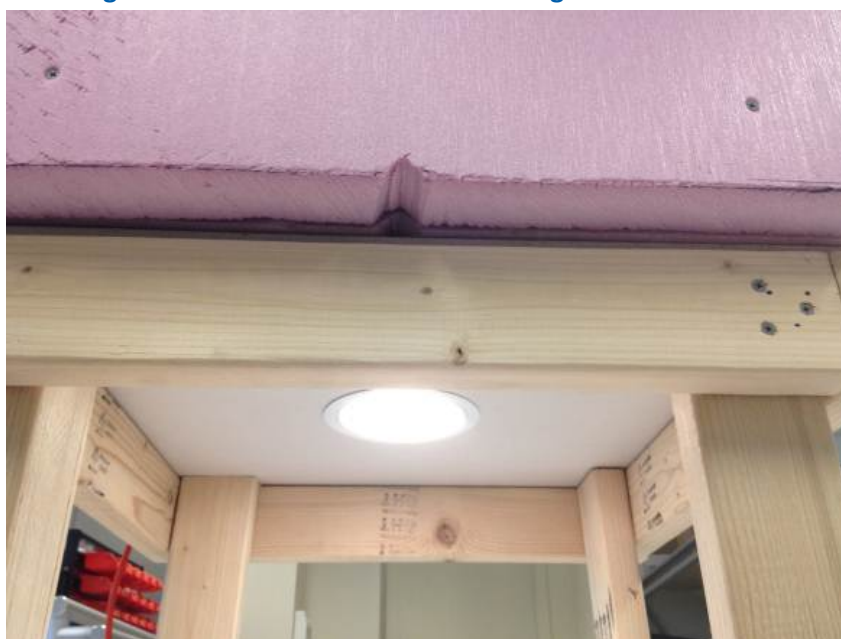
Figure HA-2. View From Below Showing Recessed Fixture
