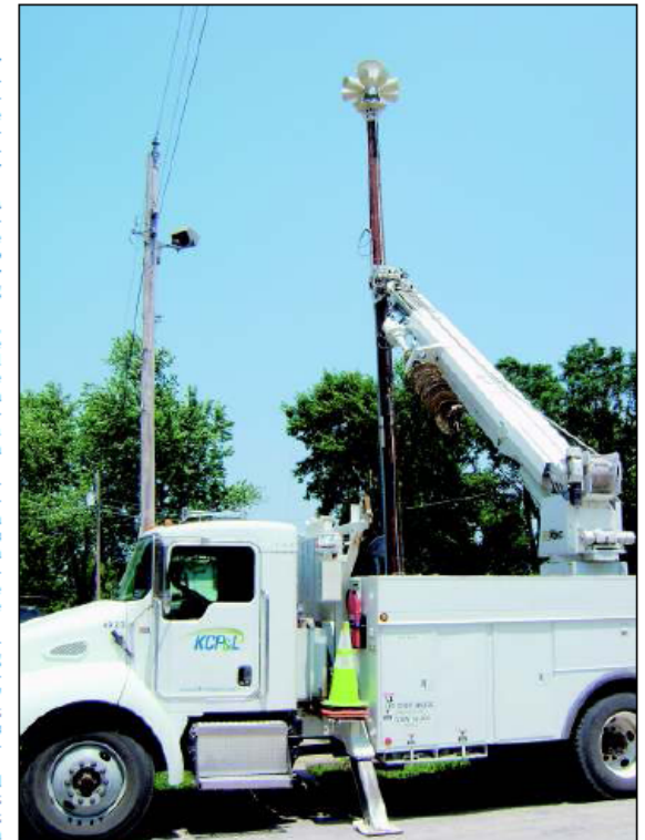
Several area communities have installed or will install new storm warning sirens this year as part of a federally funded project administered by the Northwest Missouri Regional Council of Governments. Pictured is the new siren in Pickering, which was recently placed atop its pole by crewmen from the Kansas City Power & Light Co.
