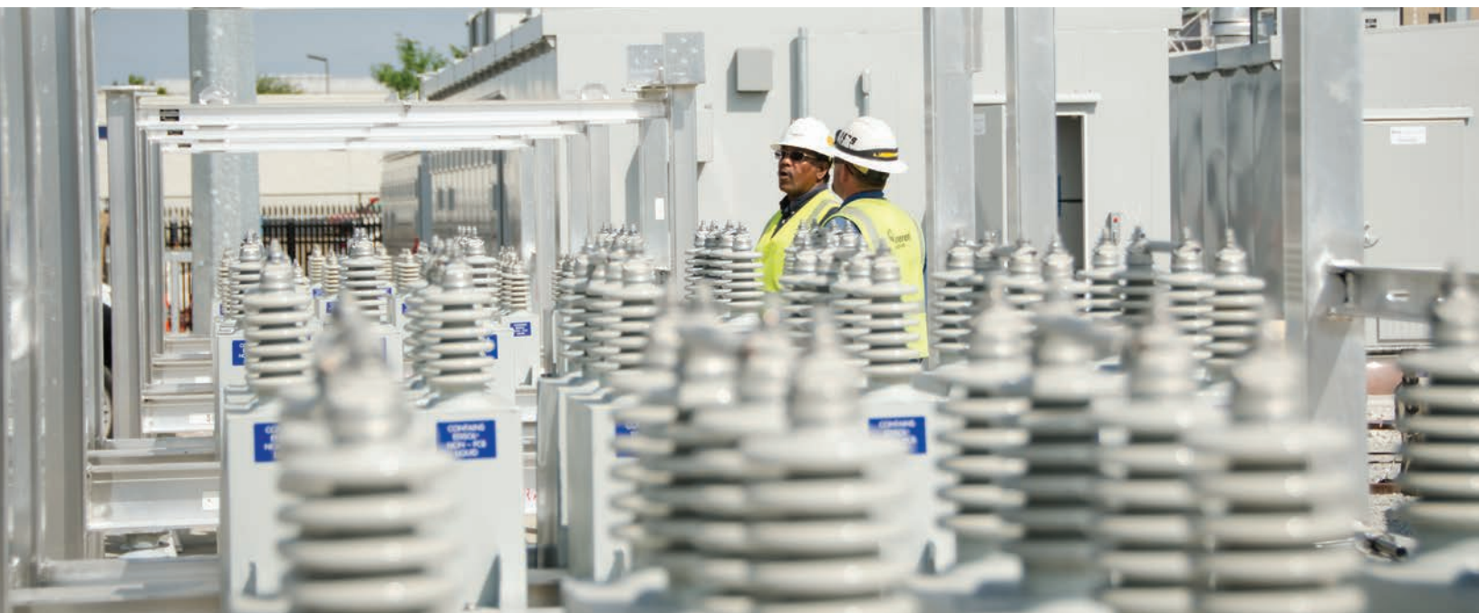
Martin Luther King substation.
