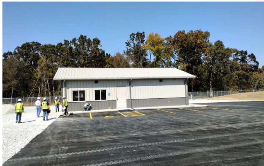
Picture 2. Walkdown and punchlist identification of the satellite O&M facility to prepare for November turnover.
