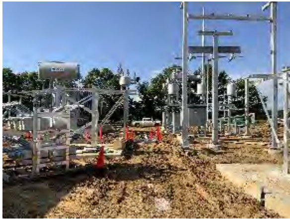
Figure 8.1: Substation Looking North
