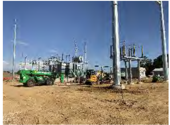
Figure 8.2: Substation Looking Southeast
