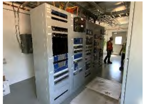
Figure 8.10: Substation Networking Controls
