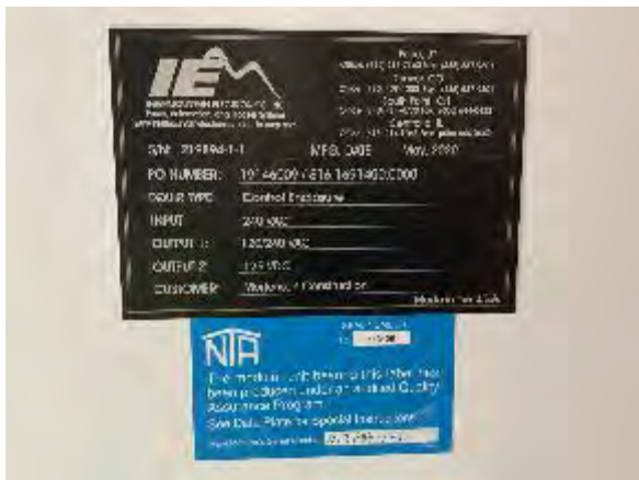
Figure 8.9: Substation Control Building Nameplate
