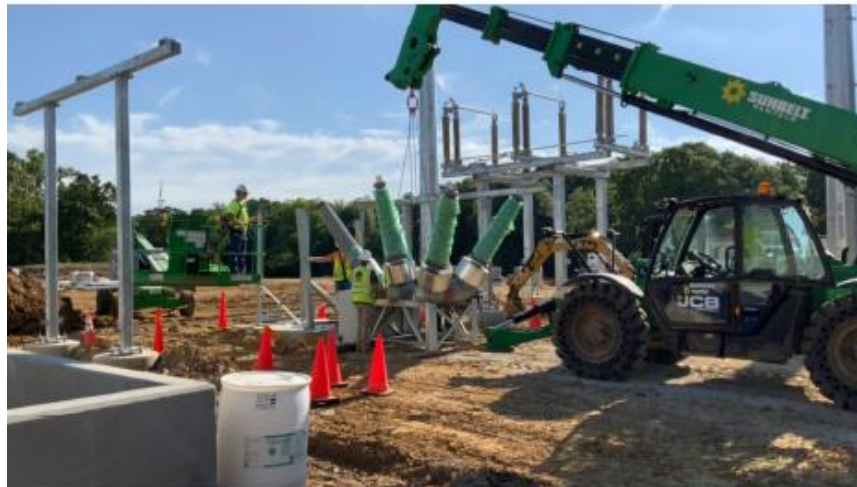
Picture 2. Preparing to install a gas-insulated circuit breaker at the collector substation.
