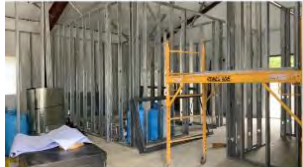
Figure 10.2: O&M Building Interior
