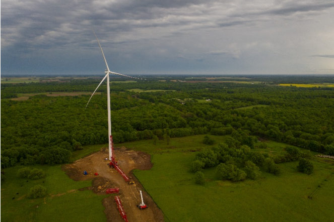
Turbine 94 Facing Southeast
