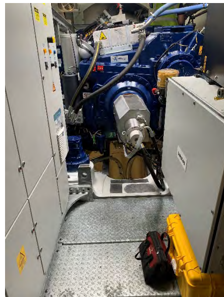
Figure 6.2: General View of Nacelle
