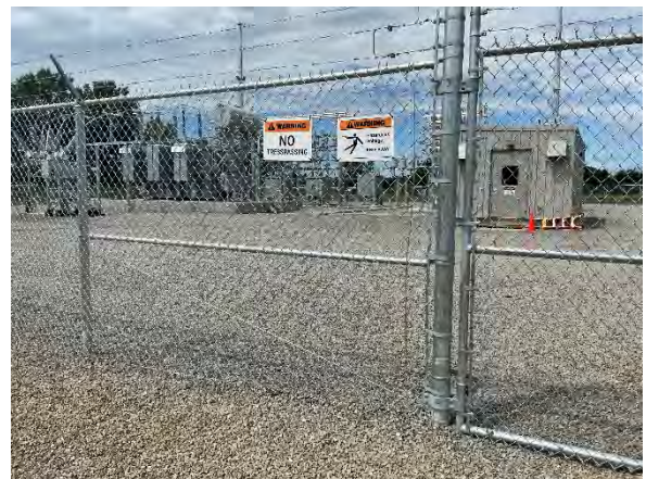
Figure 7.8: Substation Warning Signs
