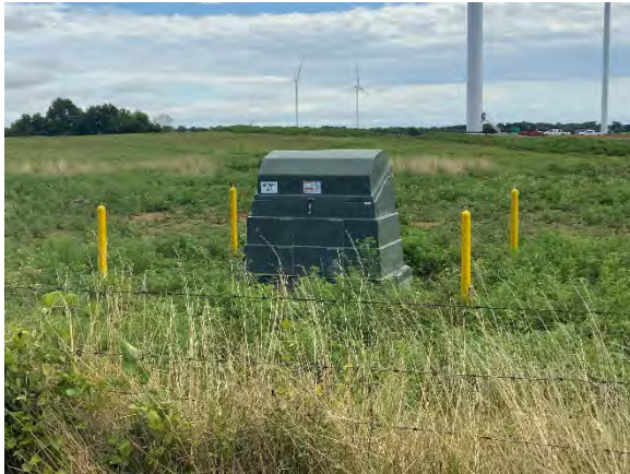
Figure 7.1: Junction Box 12A-1 12A
