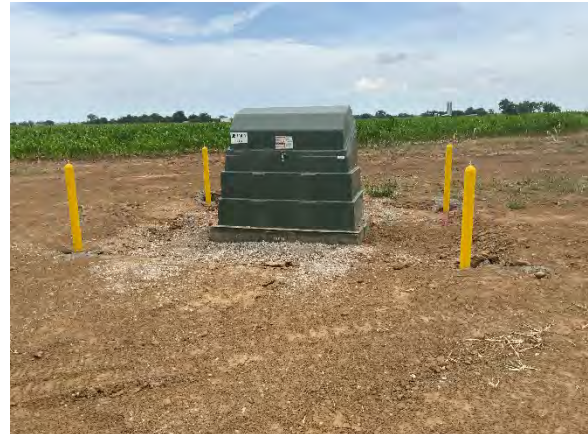
Figure 7.2: Junction Box 11B-1 11B
