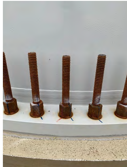
Figure 6.6: T-93 Anchor Bolts With Torque Marks
