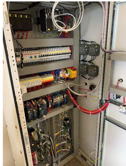
Figure 6.8: Cabinet Inside T-93 Base Section
