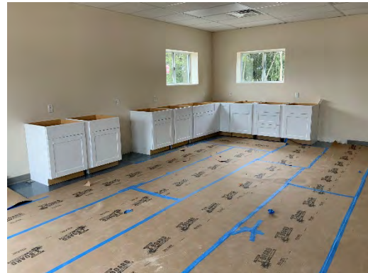
Figure 10.2: O&M Building Interior
