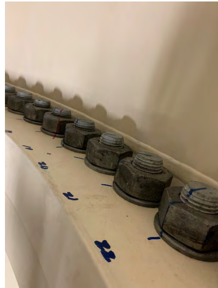
Figure 6.6: Mid Bolts With Torque Marks
