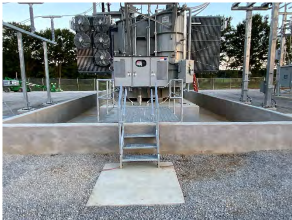
Figure 8.3: Main Power Transformer
