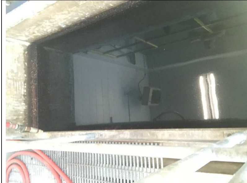
Photograph #: 005 Taken By: Zachary Miller Entity: Ironton PWS PWS ID: MO4010402 Location: Water Treatment Plant Description: Greensand Plus Media basin, not in picture but includes a 12.5% chlorine drip Date Taken: 3/1/2021 Program: PDWB
