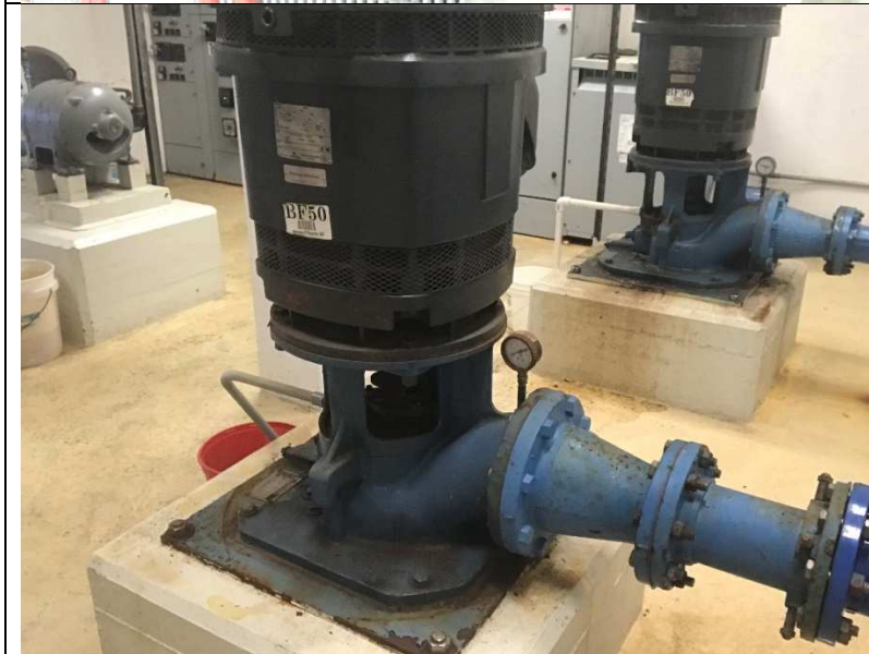
Photograph #: 006 Taken By: Zachary Miller Entity: Ironton PWS PWS ID: MO4010402 Location: Water Treatment Plant Description: High Service Pumps Date Taken: 3/1/2021 Program: PDWB
