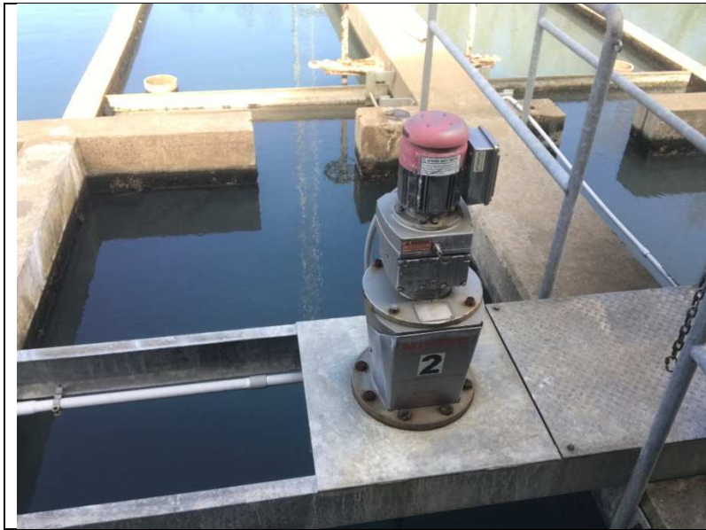
Photograph #: 004 Taken By: Zachary Miller Entity: Ironton PWS PWS ID: MO4010402 Location: Water Treatment Plant Description: Rapid Mix #2, redundant Rapid Mix #1 not pictured but looked to be in the condition. Date Taken: 3/1/2021 Program: PDWB
