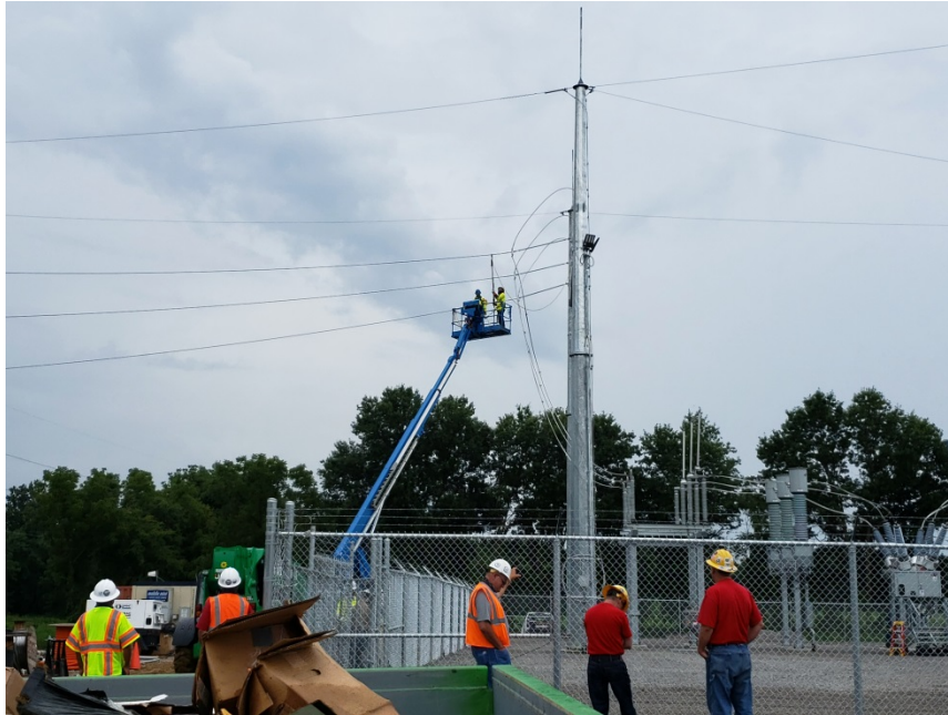
Picture 3. Line crew removing grounds from generation tie line to prepare for energization.
