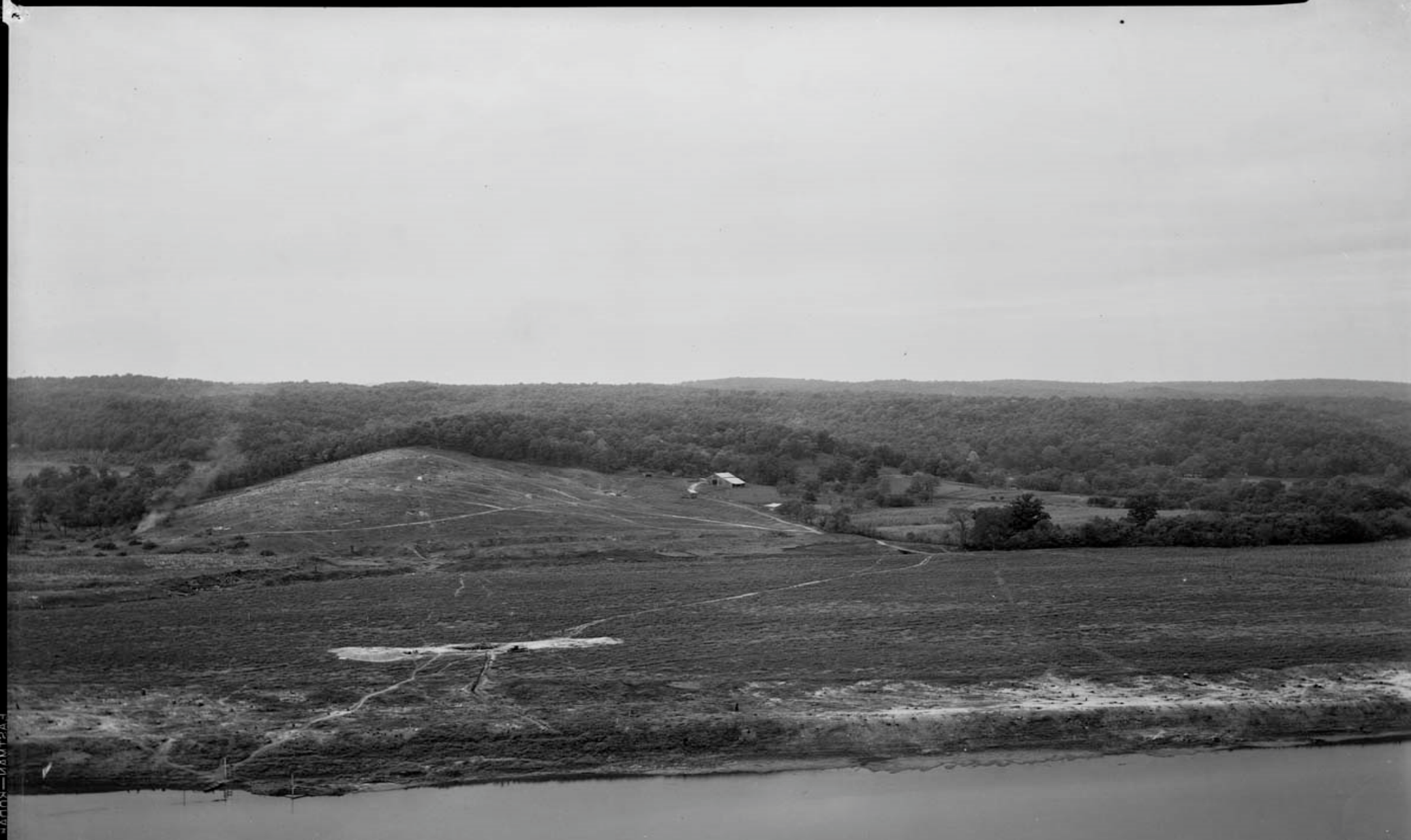
UNION ELECTRIC LIGHT & POWER CO. - HYDROELECTRIC STATION, OSAGE DEVELOPMENT STONE & WEBSTER ENGINEERING CORPORATION, Builders. J.O. 5461 # 26 9-24-29 Looking West over dam site. N1182
