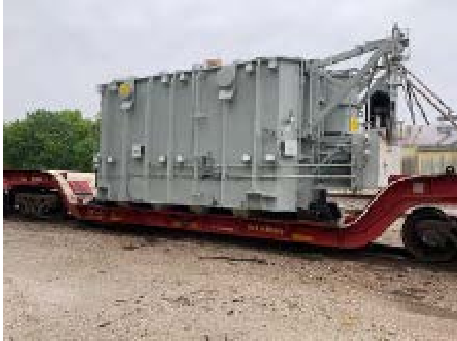
Picture 3. Main power transformer at railhead in Golden City, MO.
