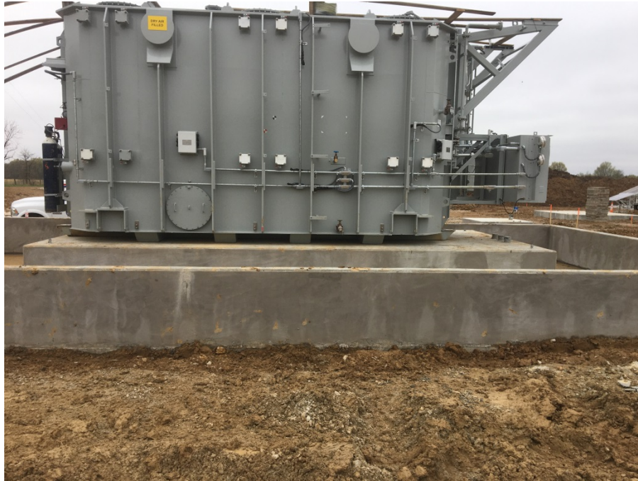
Picture 3. Main transformer on foundation (April 4, 2020).
