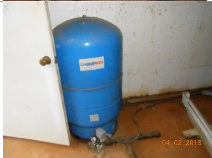
PHOTOGRAPH #2 TAKEN BY: Sheila Yoder ENTITY: Chelsea Rose Subd PERMIT: MO3031244 LOCATION: wellhouse for well#2 DESCRIPTION: bladder tank DATE TAKEN: April 2, 2018 PROGRAM: Public Drinking Water Branch
