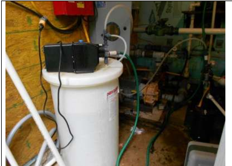
Location: Eagle Woods Subdivision Photographer: Darrell Barber Photograph Date: June 11, 2014 Comments: Chem-Tech (Series 200) chemical feed pump, 25-gallon chlorine solution tank and related piping.
