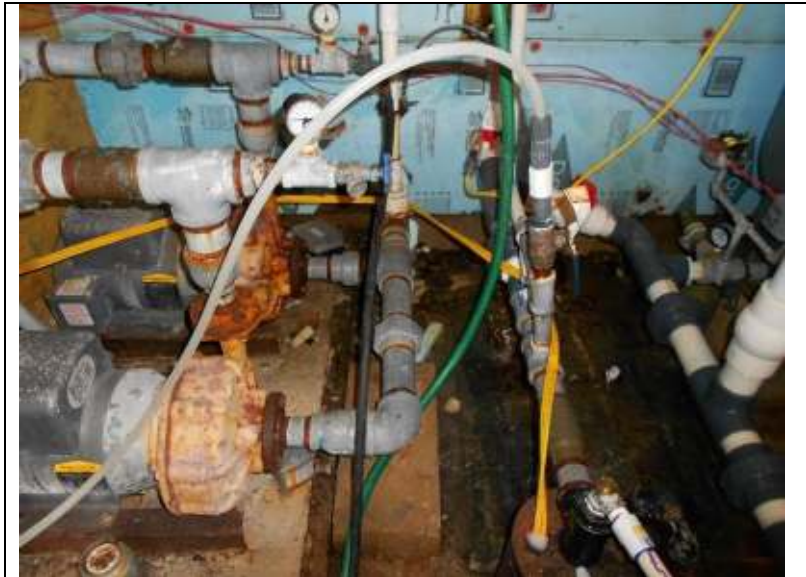
Location: Eagle Woods Subdivision Photographer: Darrell Barber Photograph Date: June 11, 2014 Comments: Booster pumps (5-hp) and related piping.
