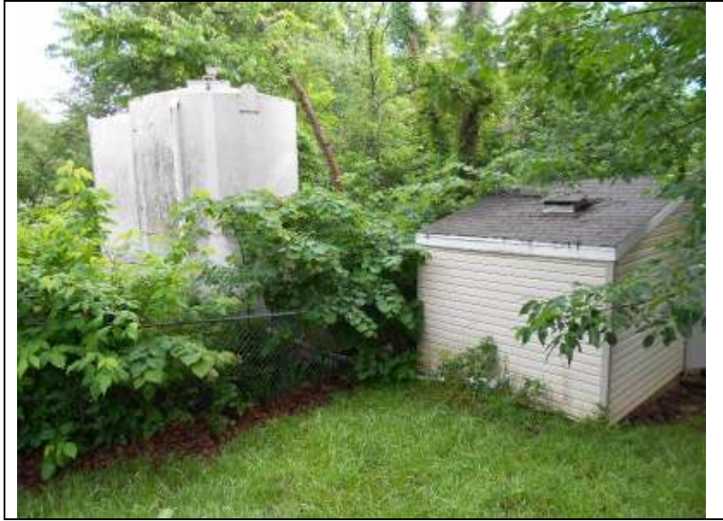
Location: Eagle Woods Subdivision Photographer: Darrell Barber Photograph Date: June 11, 2014 Comments: Well house and two 4,500-gallon ground storage tanks.
