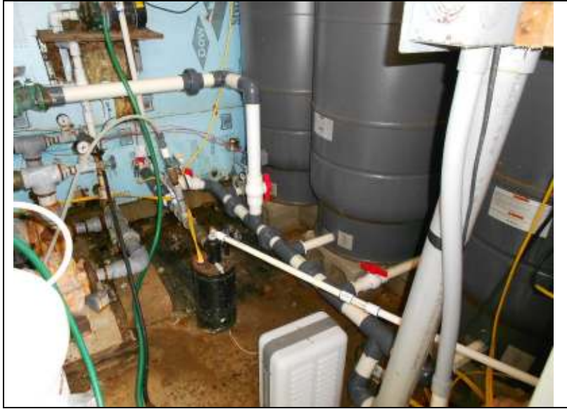
Location: Eagle Woods Subdivision Photographer: Darrell Barber Photograph Date: June 11, 2014 Comments: Well, three 119-gallon bladder tanks and related piping.
