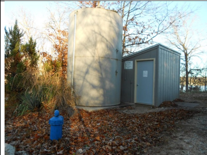
PHOTOGRAPH# 1 TAKEN BY: Darrell Barber ENTITY: Makalu Estates PERMIT: MO3031208 LOCATION: Next to well #2 facing Northwest DESCRIPTION: Well #2, 3,500-gallon ground storage tank and well house. DATE TAKEN: December 1, 2017 PROGRAM: Public Drinking Water Branch
