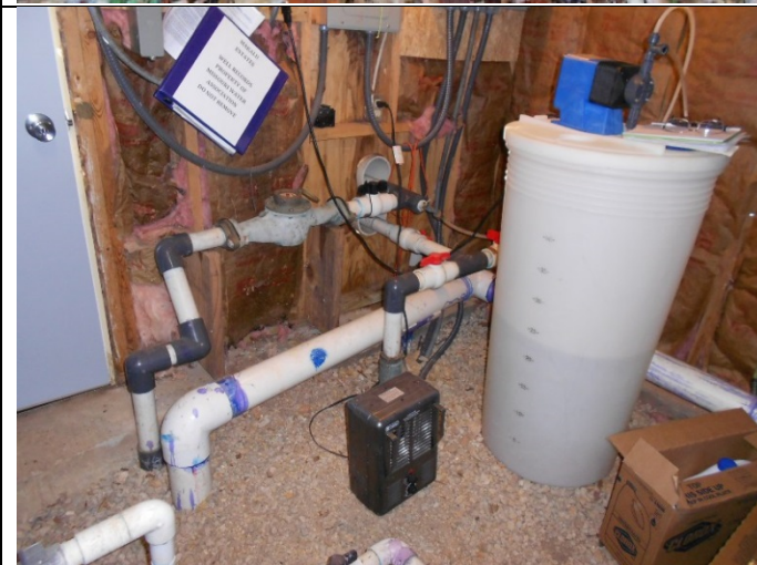
PHOTOGRAPH# 3 TAKEN BY: Darrell Barber ENTITY: Makalu Estates PERMIT: MO3031208 LOCATION: Inside well house DESCRIPTION: Chlorination system and related piping. DATE TAKEN: December 1, 2017 PROGRAM: Public Drinking Water Branch
