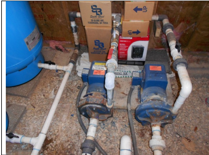
PHOTOGRAPH# 4 TAKEN BY: Darrell Barber ENTITY: Makalu Estates PERMIT: MO3031208 LOCATION: Inside well house DESCRIPTION: Two 5-hp booster pumps and related piping. DATE TAKEN: December 1, 2017 PROGRAM: Public Drinking Water Branch
