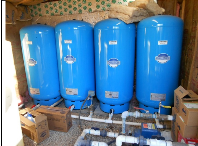
PHOTOGRAPH# 5 TAKEN BY: Darrell Barber ENTITY: Makalu Estates PERMIT: MO3031208 LOCATION: Inside well house DESCRIPTION: Four 119-gallon bladder tanks and related piping. DATE TAKEN: December 1, 2017 PROGRAM: Public Drinking Water Branch
