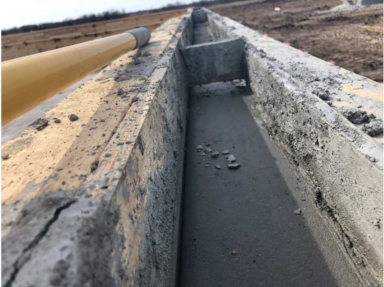
Containment wall of Main Power Transformer
