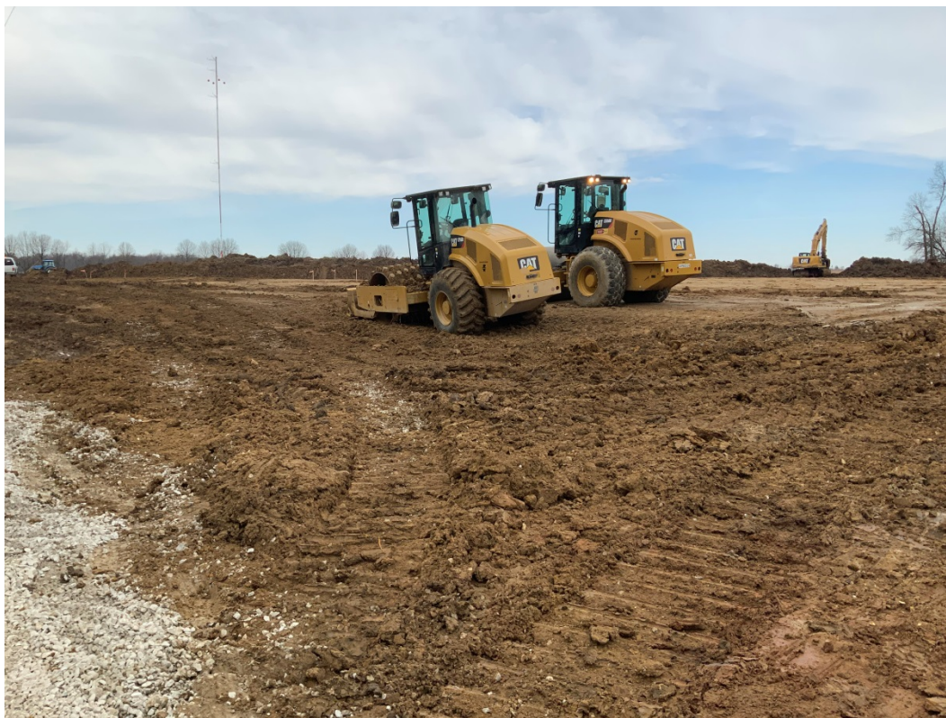
Picture 4. Mobile equipment at substation site (met tower in background left).
