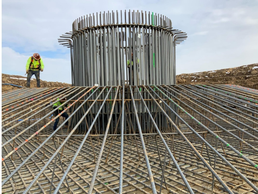
Picture 3. Complete foundation reinforcing with both rebar mats and anchor bolt cage.
