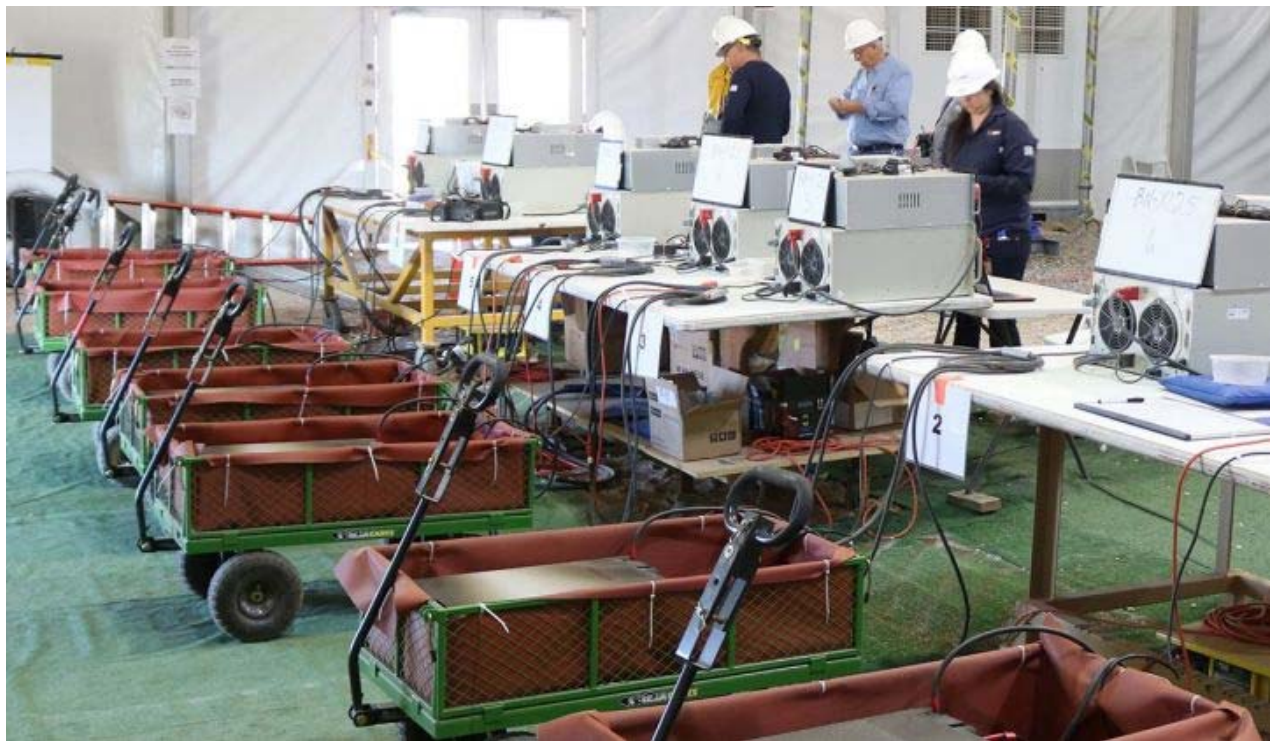
Technicians emptying out the battery modules they removed from the site of the fire. (Credit: APS)
