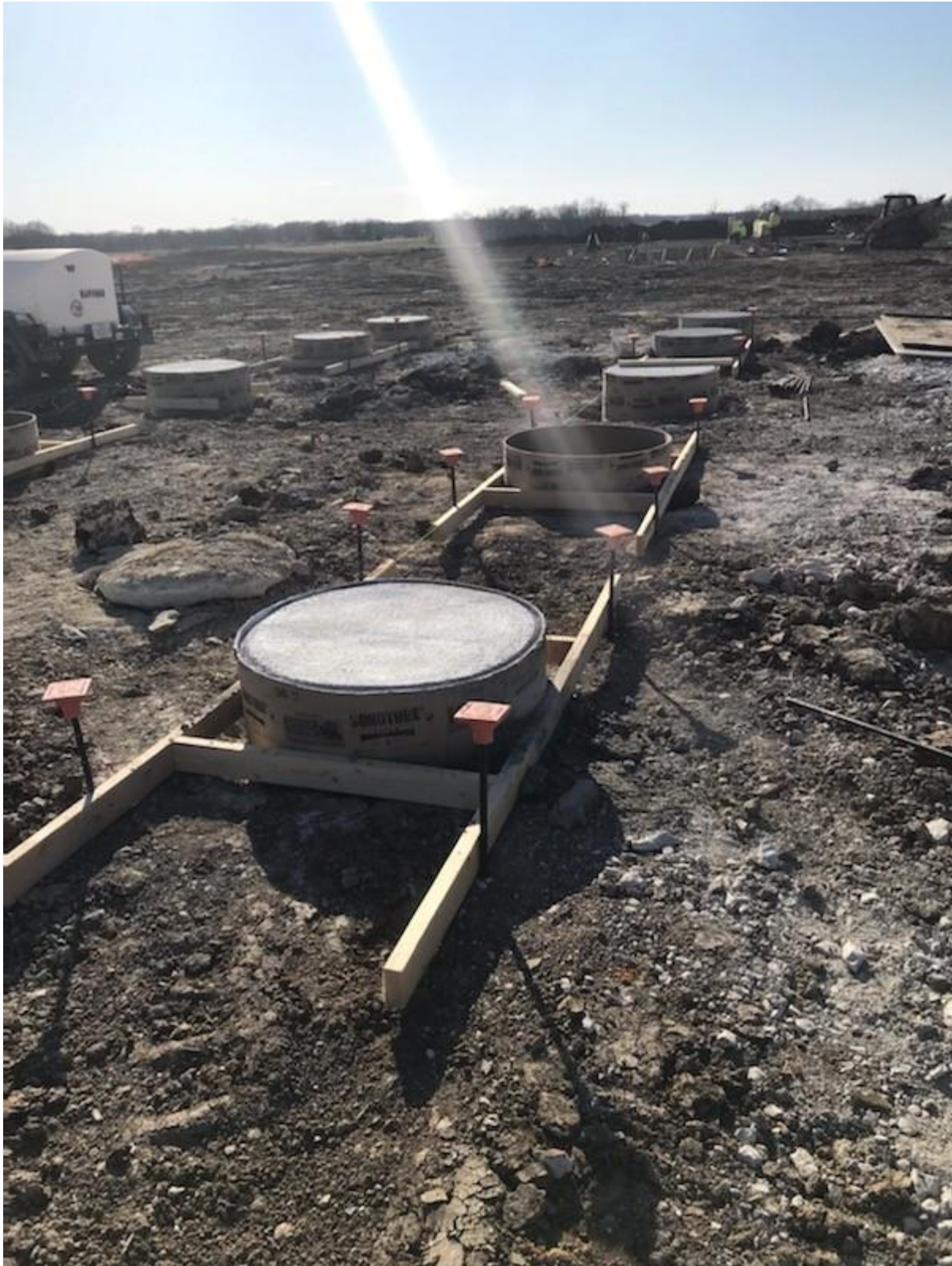
Substation Pier Foundation
