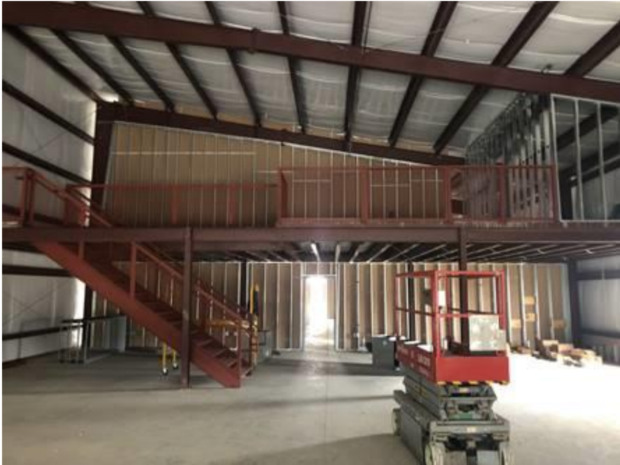
O&M Building (Interior)
