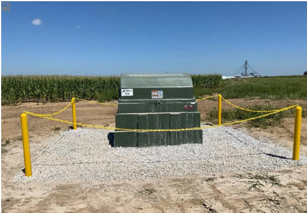
Picture 2. Bollards installed for protection of collection system junction box.
