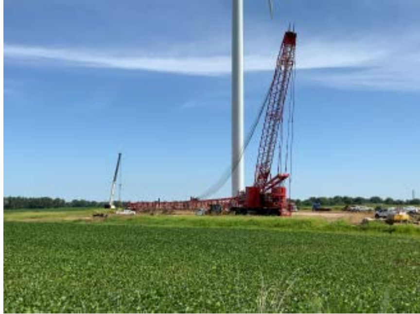
Picture 3. Main erection crane being disassembled for transfer to Kings Point project site.
