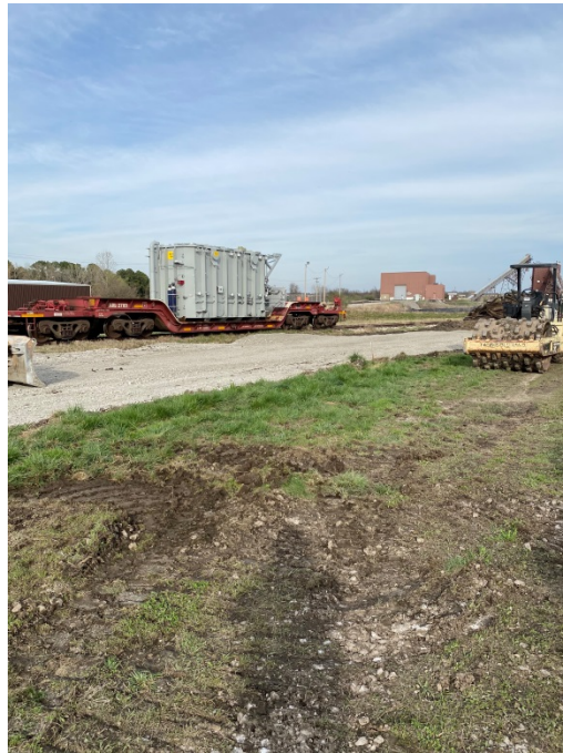
Picture 1. Main power transformer on railcar at Asbury Power Plant.
