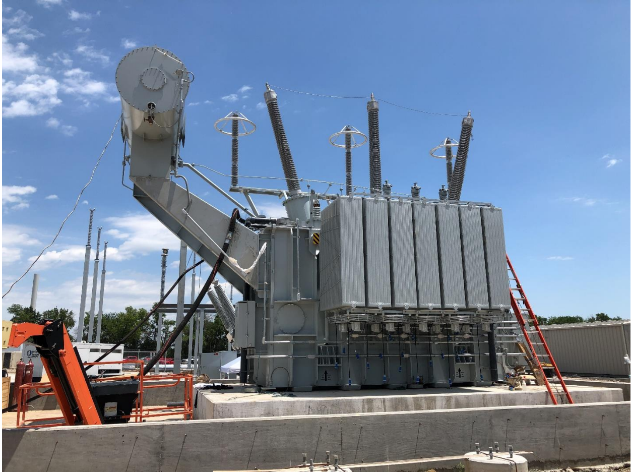
Main Power Transformer #2
