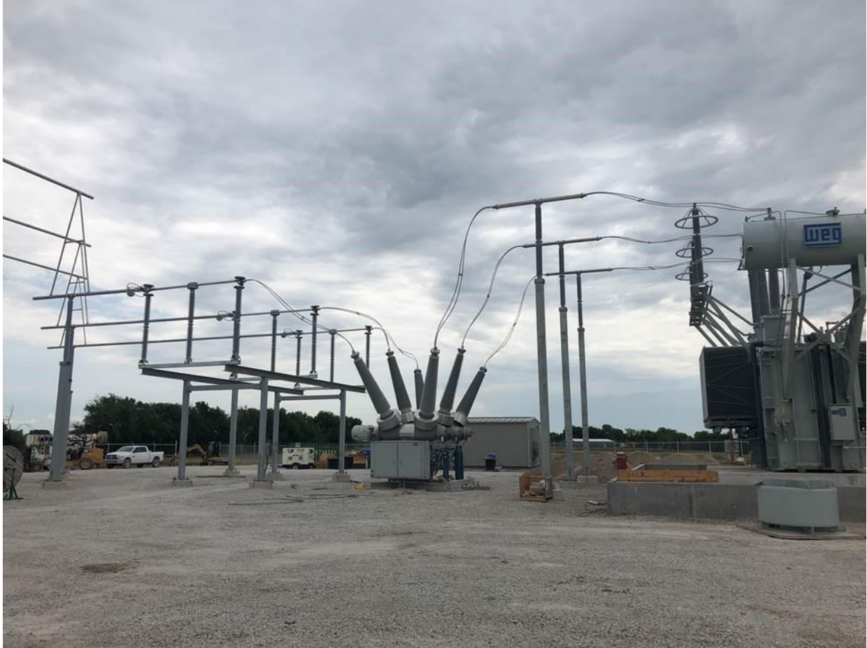
Main Power Transformer #1, Switches and Buss
