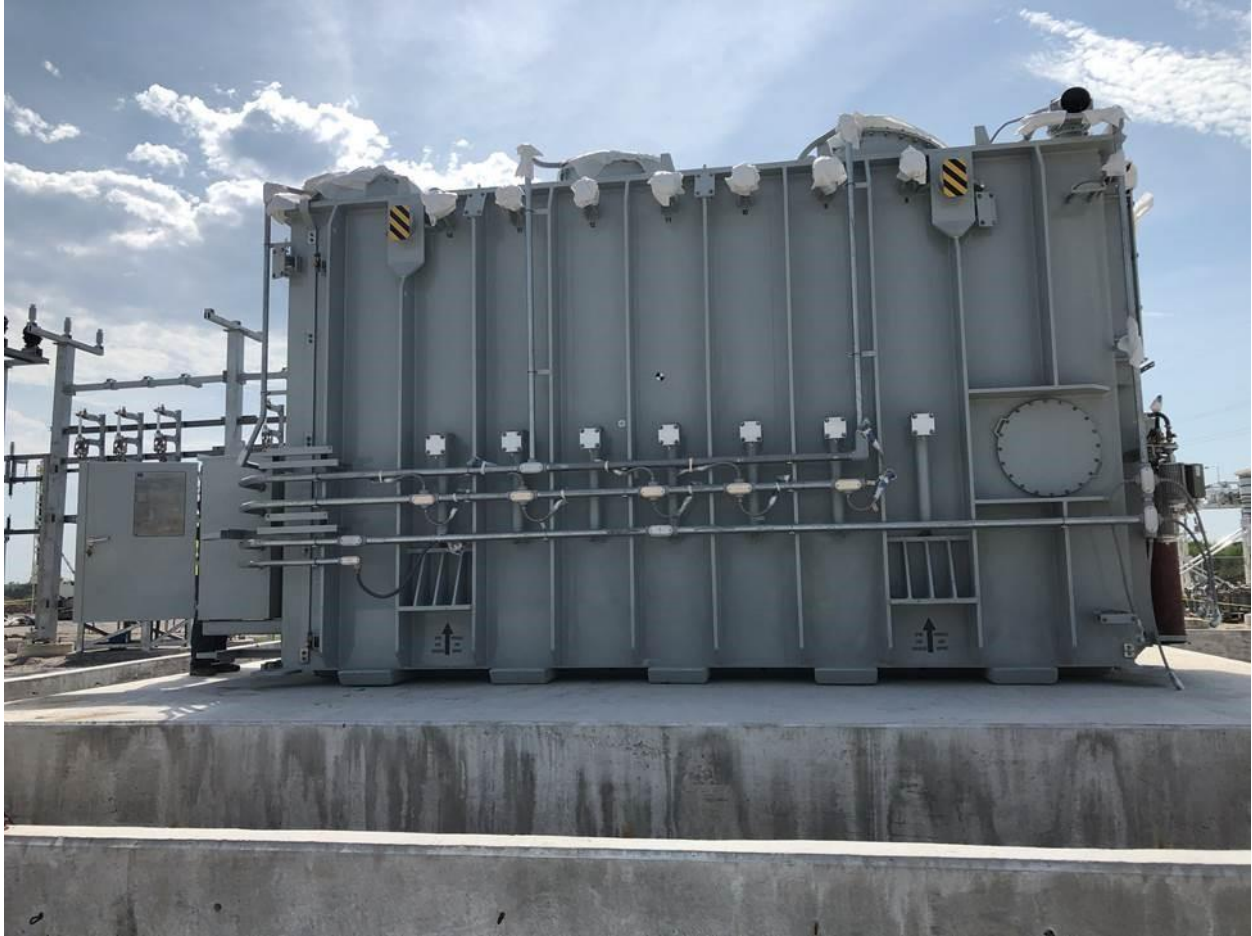
Main Power Transformer #2
