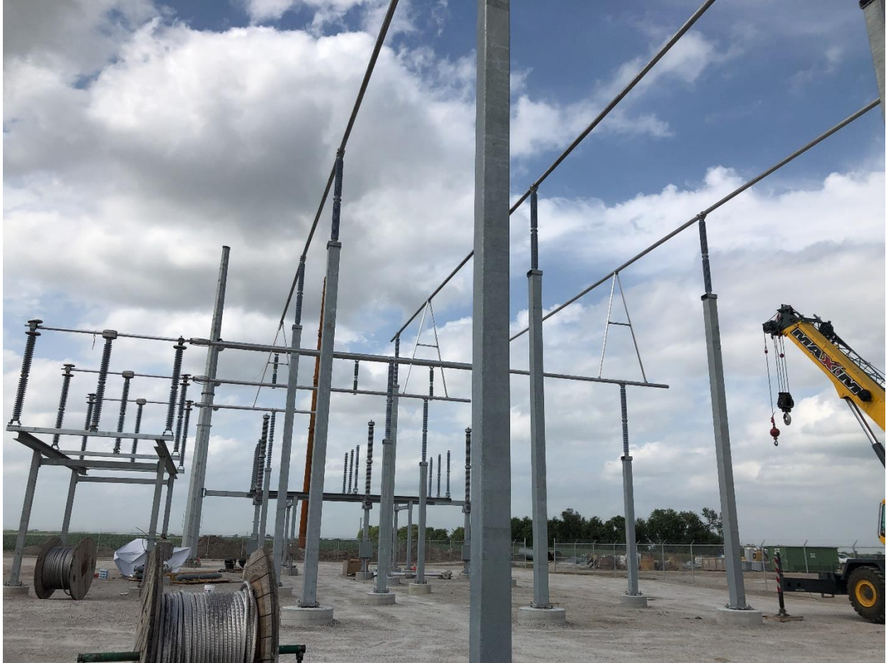
Structural Steel in Substation Yard
