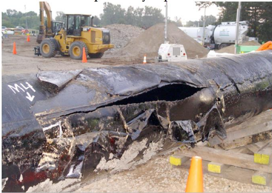
Figure 4 ERW Longitudinal Failure 15
