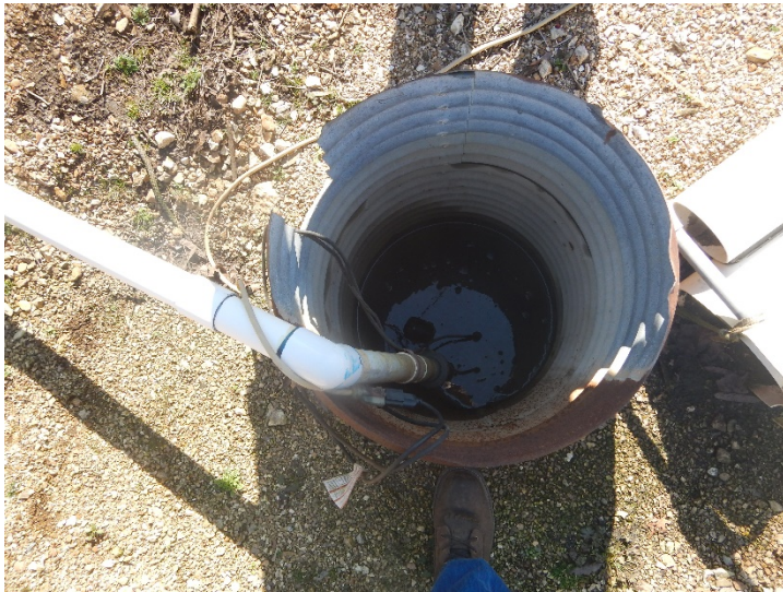
Photograph: #16 Taken By: Keith Forck Entity: Central Field Operations Permit: MOGD00340 Location: OWC KK WWTP
