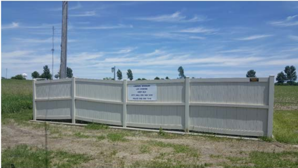
A View of the North U.S. Highway 69 Lift Station Looking East
