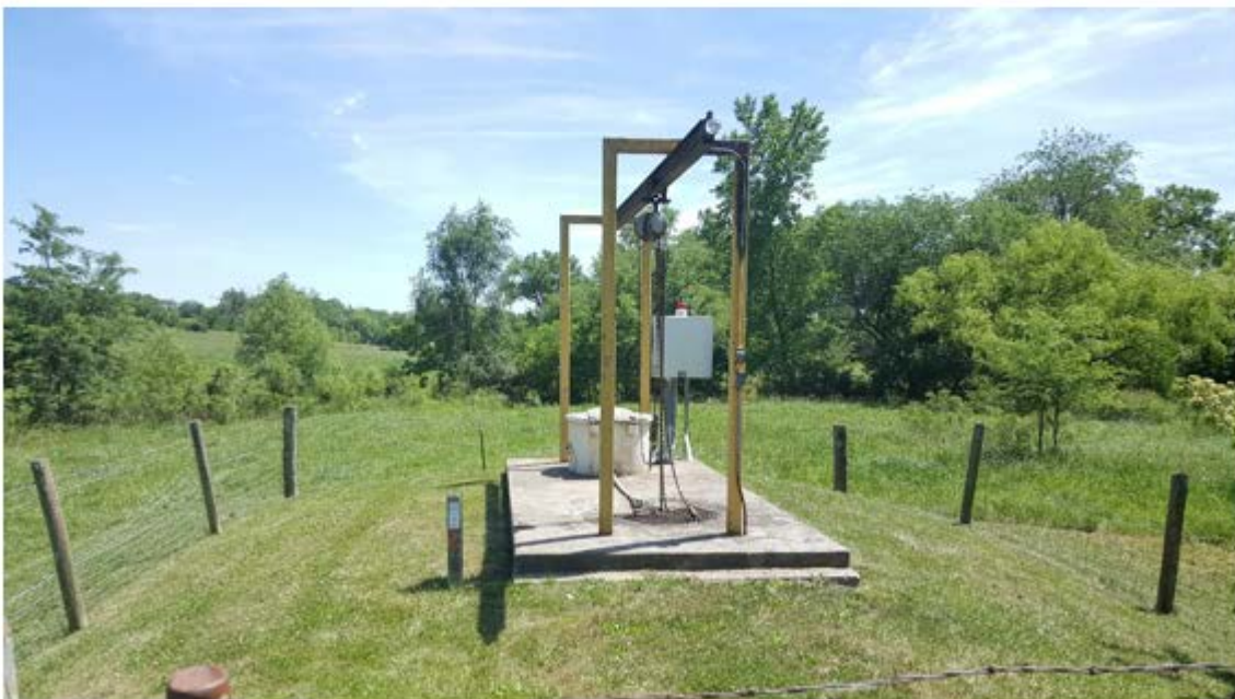
The Lift Station Located on the Schwarz Property Looking South
