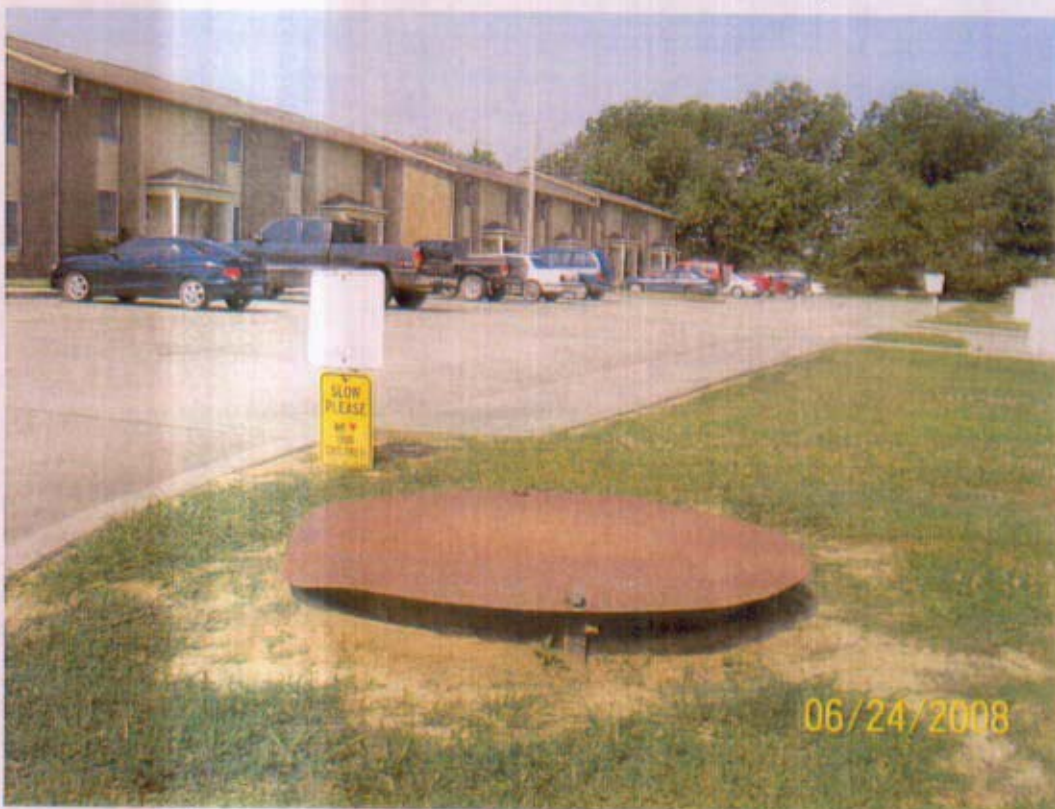
Lift Station at Westbridge Apartments.
