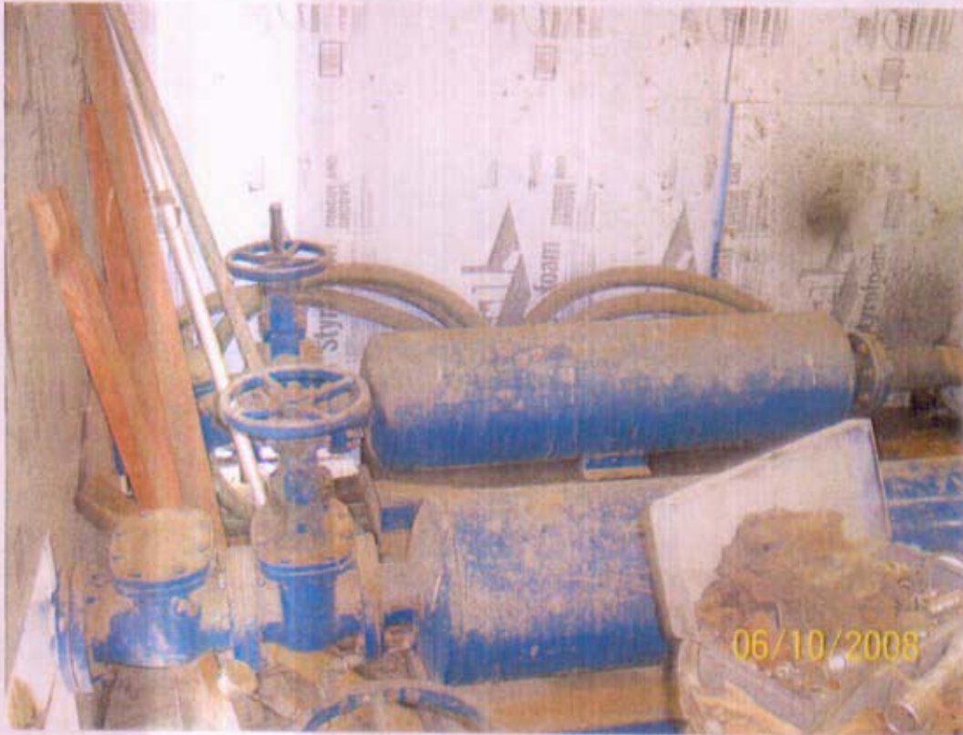
View of Blower Valve Controls
