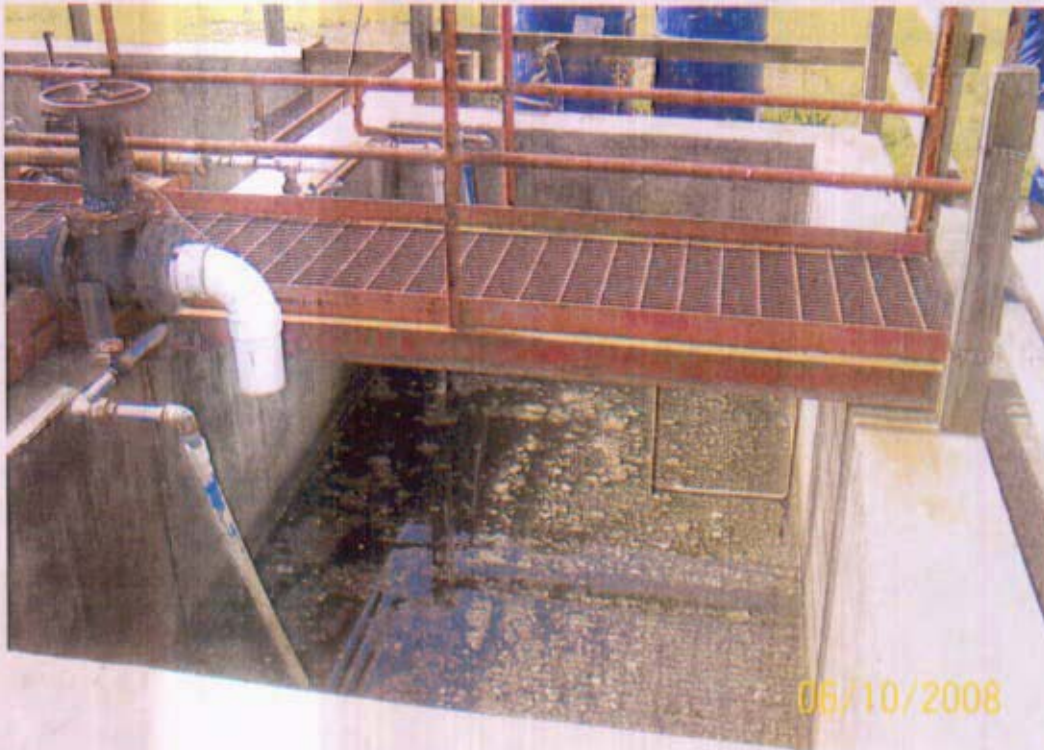
View of Waste Collection / Sludge Basin
