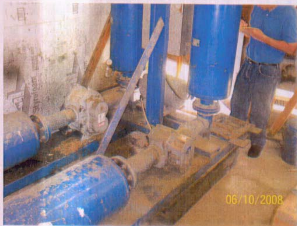
View of Motors that run Blowers
