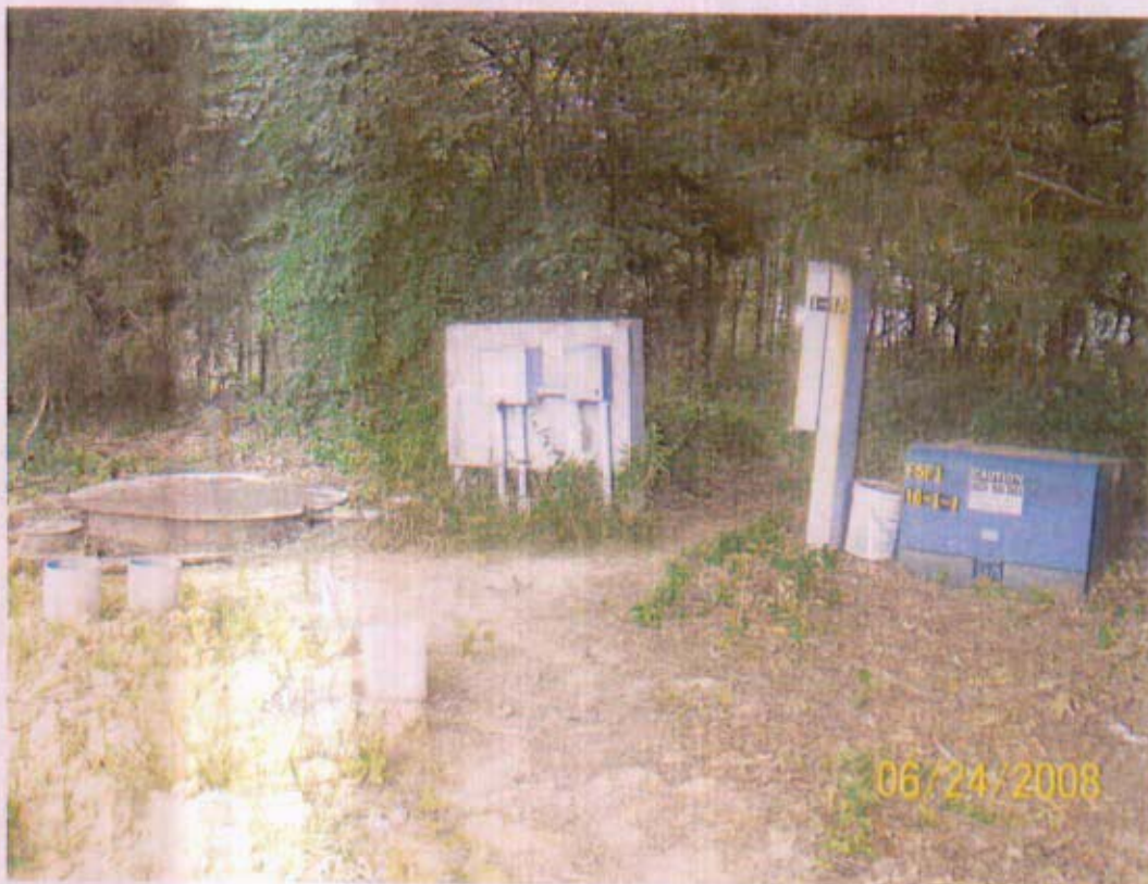
Lift Station near Intersection of Two-Mile Road and Henry Street
