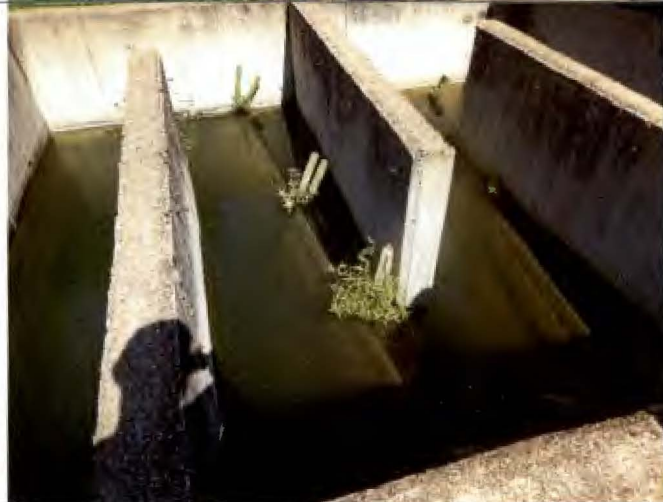
Photograph #: 006 Taken by: Wesley Hargraves Entity: Terre Du Lac Oxidation Ditch Permit: MO0095311 Location: St. Francois County
