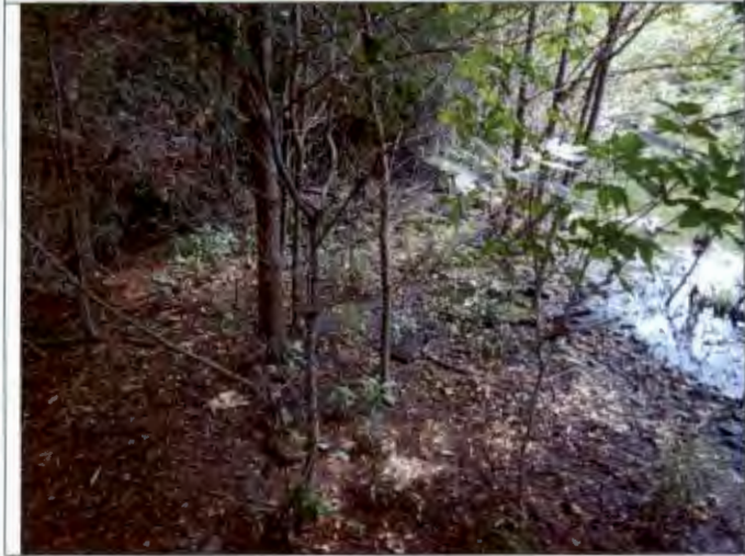
Photograph #: 015 Taken by: Wesley Hargraves Entity: Terre Du Lac North - Three Cell Lagoon Permit: MO0035700 Location: St. Francois County Description: View of the berm between the holding basin and the 2 nd cell of the old lagoon. Water levels had lowered by the time the Department arrived on site. Taken facing east. Date Taken: July 23, 2019 Program: WPC Unit
