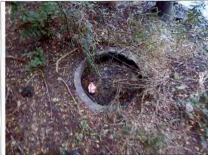
Photograph #: 016 Taken by: Wesley Hargraves Entity: Terre Du Lac North - Three Cell Lagoon Permit: MO0035700 Location: St. Francois County Description: View of manhole between 1 st and 2 nd cells of the old lagoon. Date Taken: July 23, 2019 Program: WPC Unit
