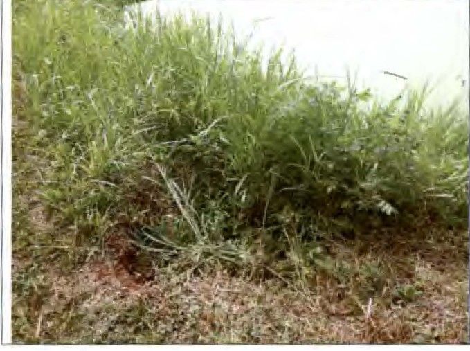
Photograph #: 003 Taken by: Wesley Hargraves Entity: Terre Du Lac South - One Cell Lagoon Permit: MO0057312 Location: St. Francois County Description: View of berm damage. Taken facing northeast. Date Taken: July 10, 2019 Program: WPC Unit
