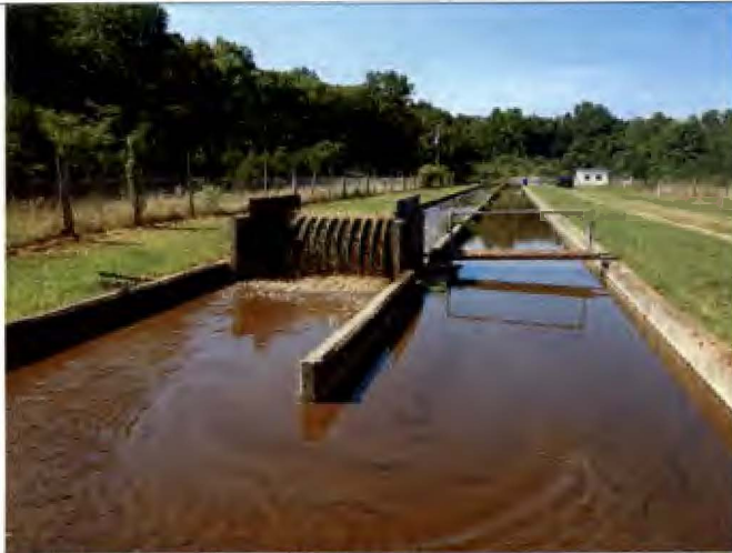
Photograph #: 001 Taken by: Wesley Hargraves Entity: Terre Du Lac Oxidation Ditch Permit: MO0095311 Location: St. Francois County Description: View of oxidation ditch and northern rotor. Taken facing south. Date Taken: July 10, 2019 Program: WPC Unit
