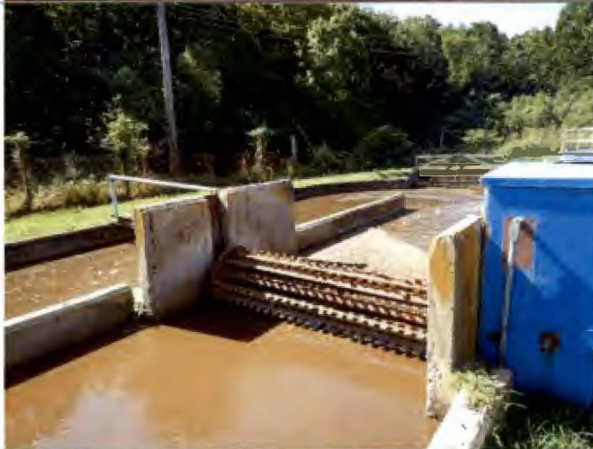
Photograph #: 002 Taken by: Wesley Hargraves Entity: Terre Du Lac Oxidation Ditch Permit: MO0095311 Location: St. Francois County Description: View of southern rotor. This rotor was not operable at the time of the inspection. Taken facing south. Date Taken: July 10, 2019 Program: WPC Unit
