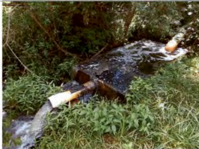
Photograph #: 006 Taken by: Wesley Hargraves Entity: Terre Du Lac North - Three Cell Lagoon Permit: MO0035700 Location: St. Francois County Description: View of Outfall #001. Taken facing southeast. Date Taken: July 10, 2019 Program: WPC Unit
