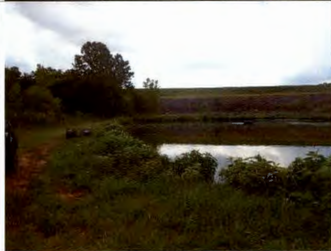
Photograph #: 002 Taken by: Wesley Hargraves Entity: Terre Du Lac North - Three Cell Lagoon Permit: MO0035700 Location: St. Francois County Description: View of primary cell and broken aerator. Taken facing southeast. Date Taken: July 10, 2019 Program: WPC Unit
