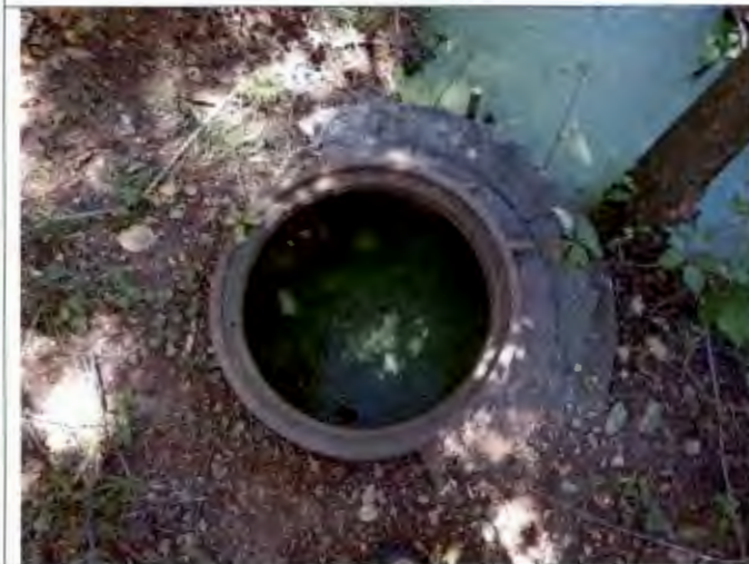
Photograph #: 018 Taken by: Wesley Hargraves Entity: Terre Du Lac North - Three Cell Lagoon Permit: MO0035700 Location: St. Francois County Description: View of manhole between 2 nd and 3 rd cells of old lagoon. Date Taken: July 23, 2019 Program: WPC Unit
