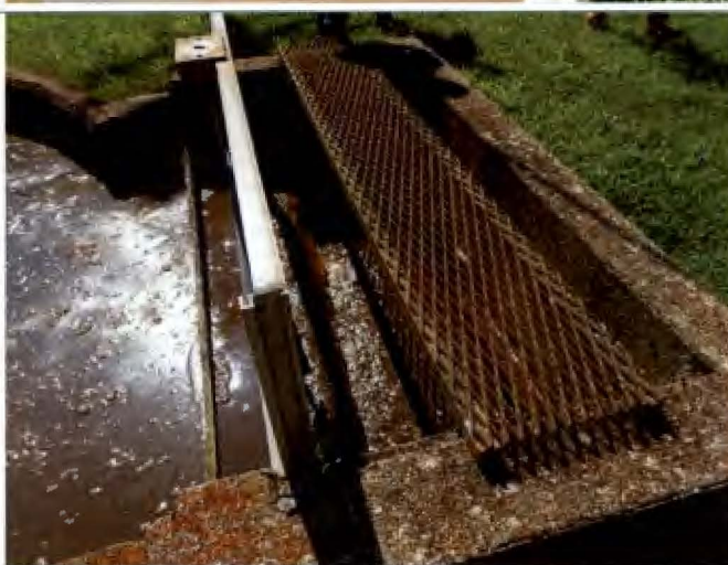
Photograph #: 003 Taken by: Wesley Hargraves Entity: Terre Du Lac Oxidation Ditch Permit: MO0095311 Location: St. Francois County Description: View of outlet box to clarifier. Taken facing southeast. Date Taken: July 10, 2019 Program: WPC Unit
