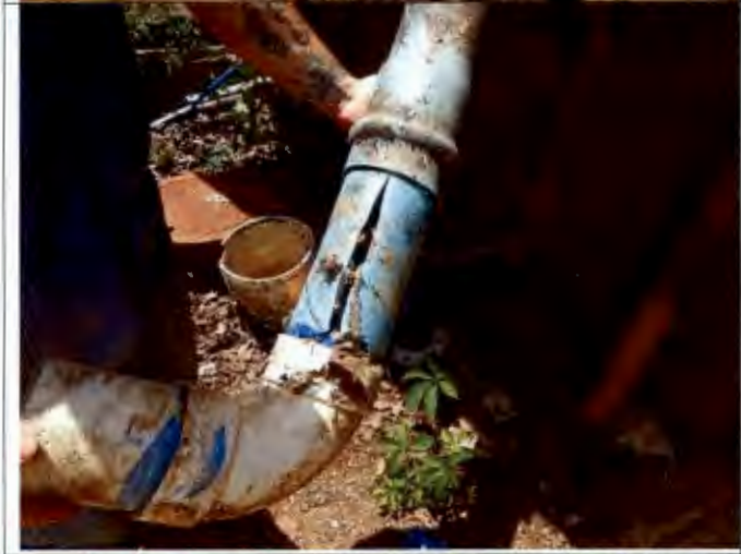
Photograph #: 014 Taken by: Wesley Hargraves Entity: Terre Du Lac North - Three Cell Lagoon Permit: MO0035700 Location: St. Francois County Description: View of damaged pipe. The cause of the overflow. Date Taken: July 23, 2019 Program: WPC Unit
