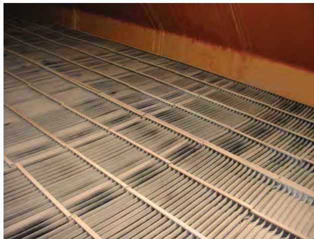
Figure 2-3 – Existing Mist Eliminators
